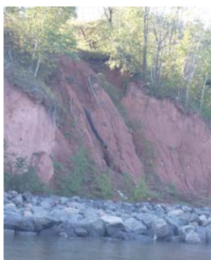
Eroding slope in front of Lighthouse
