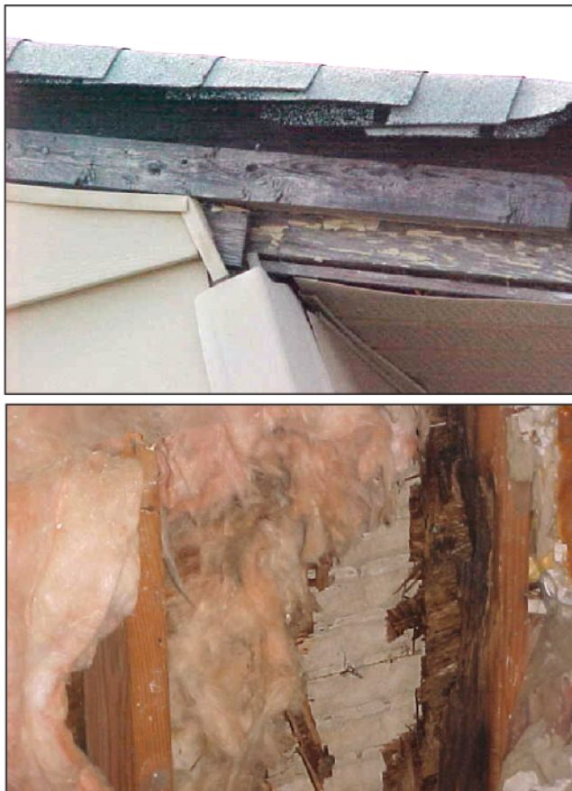
Figure 14—Results of poor maintenance: (top) damage to fascia and roof; (bottom) damage to inside of exterior walls caused by leaky plumbing.
