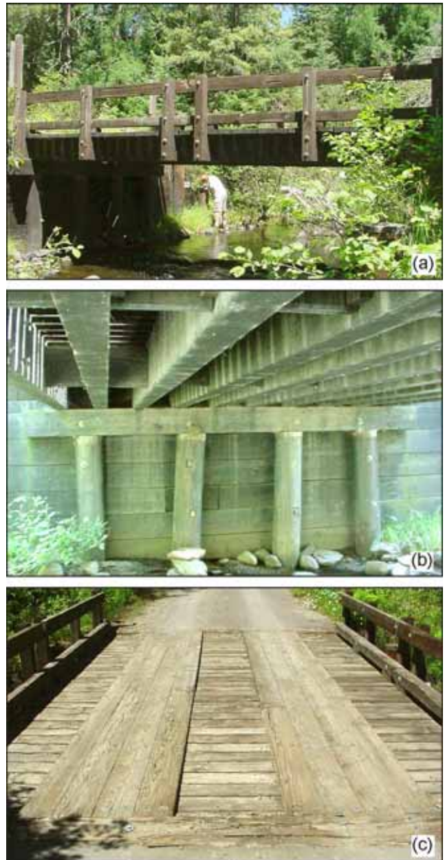
Figure 1—Typical single-span girder timber bridge: (a) side view, (b) structure, (c) deck.
