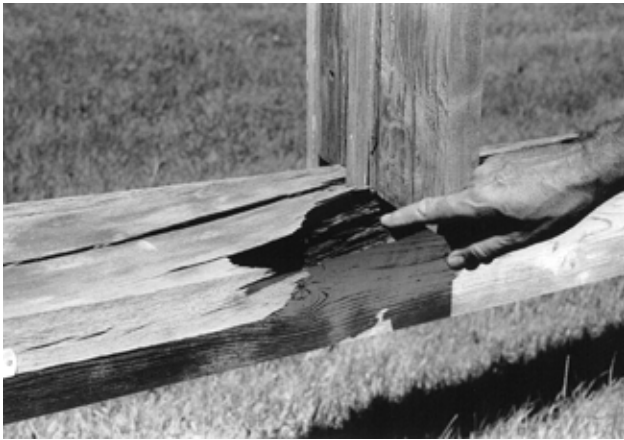
Figure 14—Decay of untreated window unit. Window unit fell apart after 6 years of outdoor exposure.
