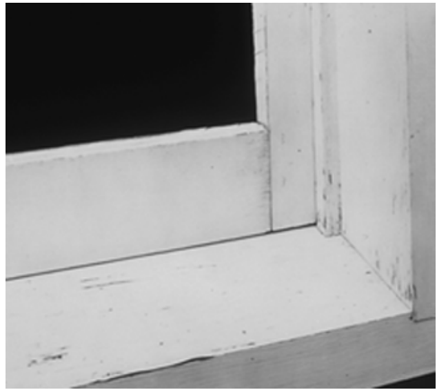
Figure 12—Window units after 5 years of exposure. Top: Sash and frame not treated before painting. Bottom: Sash dipped in WRP for 3 min before painting and WRP brushed onto frame
