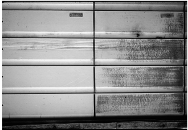
Figure 9—Black stain on wood caused by mildew.
