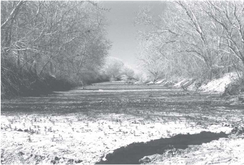
Figure 6.—The mouth of the Arroyo Pasajero, which is choked with sediment as it opens onto an impoundment basin where sediments are deposited next to the California Aqueduct.
