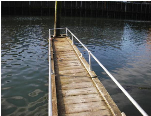
C. Galvanized pipe “bull rails”.
