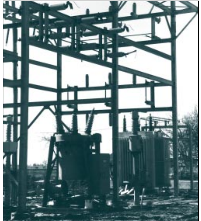
Owning their own utilities gives Shelbina flexibility for meeting the needs of citizen and businesses.
