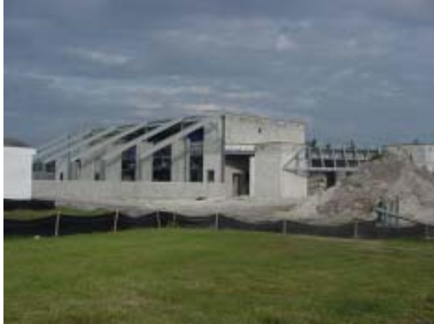
The new biological control quarantine facility is under construction at the ARS Invasive Plant Research Laboratory, Ft. Lauderdale, FL.
