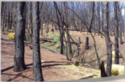
Straw is used for mulch and check dams are constructed in burned areas to stop erosion.
