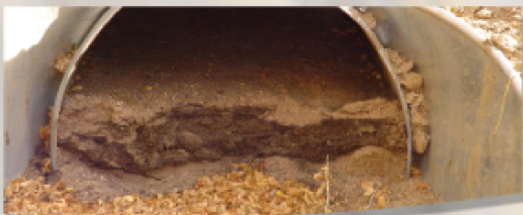
Post-fire erosion nearly fills this culvert with sediment.
