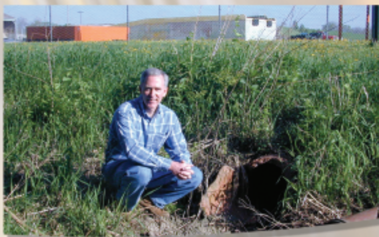
Dick Wager, Miami County Engineer's Office, manages the project that will install storm sewer collection systems to prevent pollutants from running into the Great Miami River.
