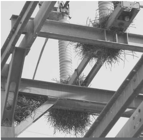
Monk parakeet nests built in electrical substations often cause power outages that result in loss of service and expensive repairs. (APHIS file photo.)
