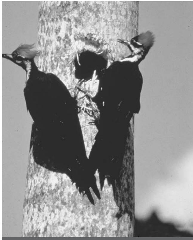
Pileated woodpeckers can cause substantial damage to utility poles. (USDA Forest Service photo by Mike Ostry.)
