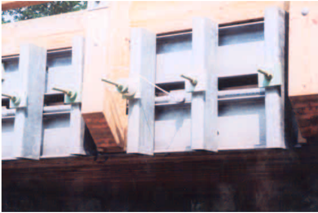
Figure 15 —Load cells were installed on stressing bars to monitor changes in bar tension.
