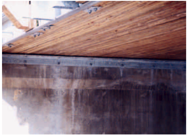
Figure 11—Superstructure was attached by bolting steel angles to sides of abutments, then bolting bridge to steel angles.
