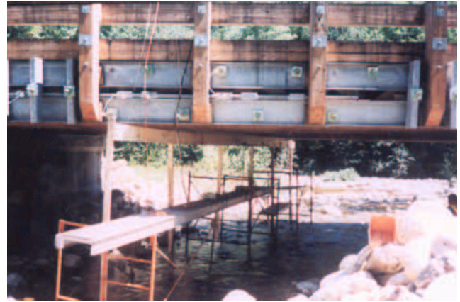
Figure 16 —Bridge deflections of load tests 1 and 2 were measured using displacement transducers attached to a wood beam supported by scaffolding.
