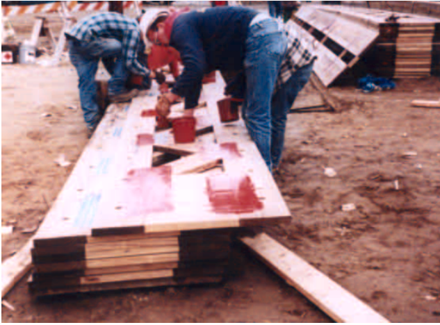
Figure 6—Brush painting of galvanized metal plate connectors of each truss at site for additional protection from corrosion.
