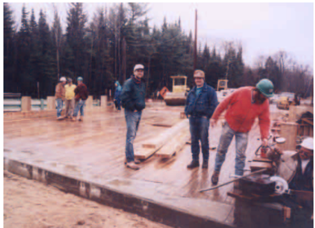
Figure 12—Bridge after construction of backwalls and installation of rail post and curb.
