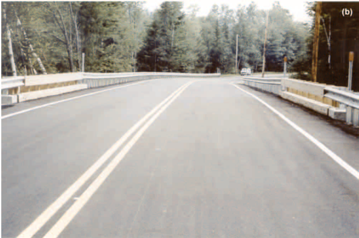
Figure 14—Completed Byron bridge: (a) profile of completed bridge (looking east); (b) completed bridge just after paving (looking south).
