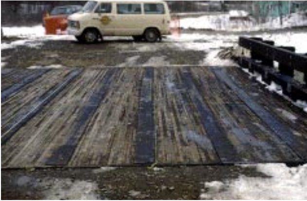
Figure 20—Slight hourglass shape was noticeable soon after initial stressing. Note stringline aligned with web member in middle of photograph.
