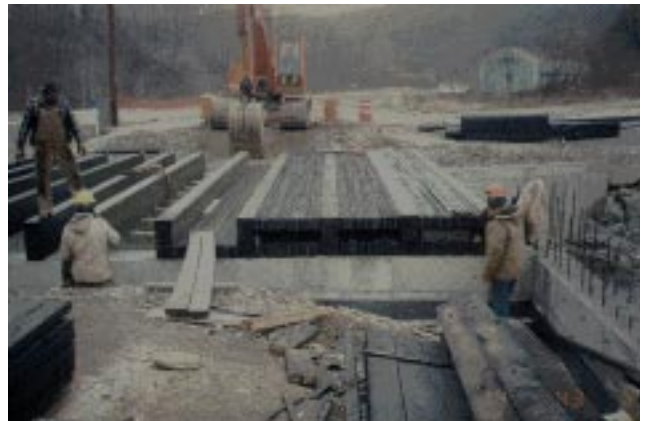
Figure 8—On-site assembly of the superstructure consisted of (top) placement of the glulam beam web members with a backhoe and nylon straps, (middle) placement of the lower flange lumber laminations by hand with standard 38- by 89-mm boards providing temporary support at the butt-joint locations, (bottom) insertion of the solid-block diaphragms at the ends of the bridge as the upper and lower flanges were completed.
