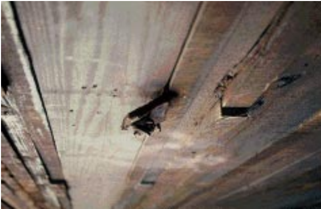
Figure 21—Cardboard corner strapping protector was not removed at installation and caused a visible separation between lower flange laminations.
