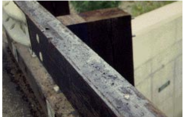
Figure 22—Excess creosote preservative was noticeable at several steel bearing plates (top) and along the top surface of the glulam timber rail (bottom).
