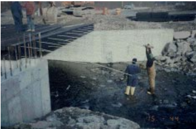
Figure 9—Full-width stressing bars were inserted into the upper and lower flanges by hand (top). When poor hole alignment prevented insertion by hand, a portable hand drill was used (bottom).
