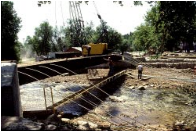
Figure 11—Placement of full-width, steel stressing bars through prebored holes in the top and bottom flanges.
