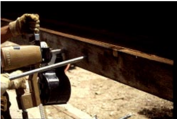
Figure 9—Preassembly of the bridge components into modules at the fabrication plant. Temporary supports were used to align members (top); temporary dowels and nails were placed to fasten members (bottom).
