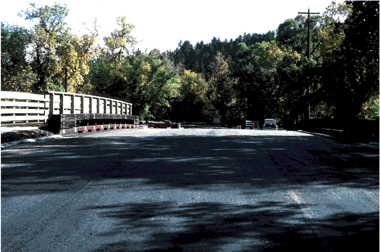
Figure 13—The completed Spearfish Creek bridge: side view (top) and end view (bottom), looking north.
