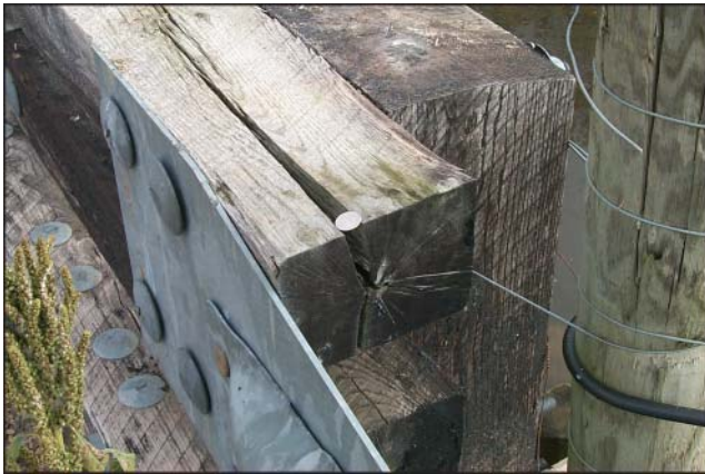
Figure 14—Large end-check and split in rail member of Laurel Run bridge (Huntingdon County).
