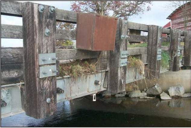
Figure 17—Significant plant growth (indicating moisture accumulation near scupper block openings) at Laurel Run bridge (Huntingdon County).
