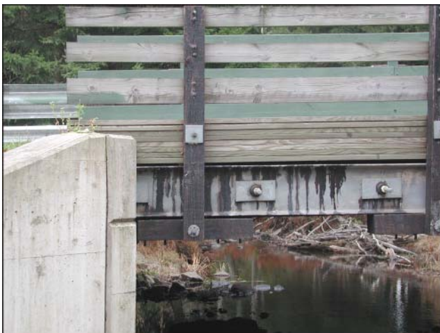
Figure 16—Noticeable creosote preservative bleeding at Birch Creek bridge.
