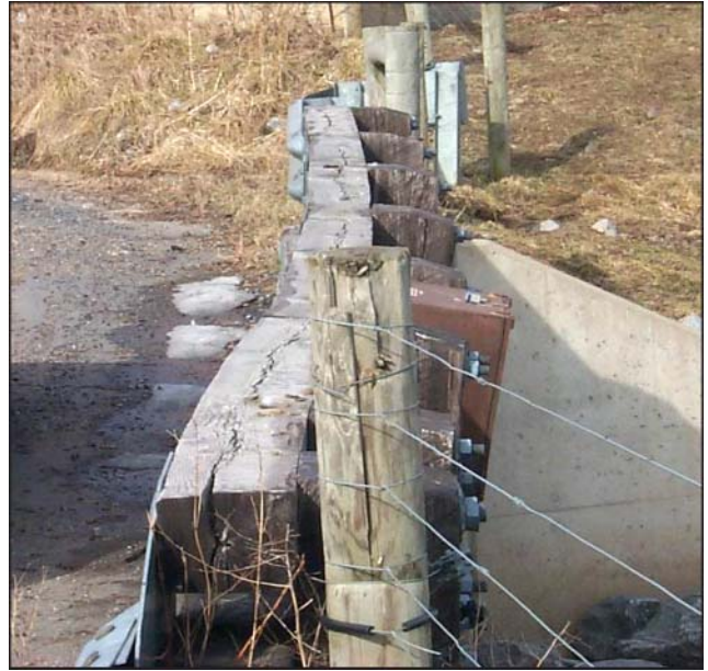
Figure 20—Large bowing of rail member at Laurel Run bridge (Huntingdon County).
