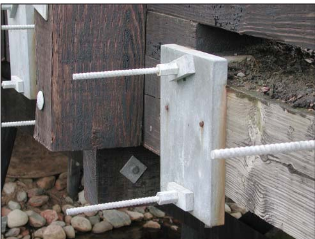
Figure 19—One alternative method to re-tension stress-laminated bridges with limited bar extension is to use external prestressing, with one bar above and one below the deck.
