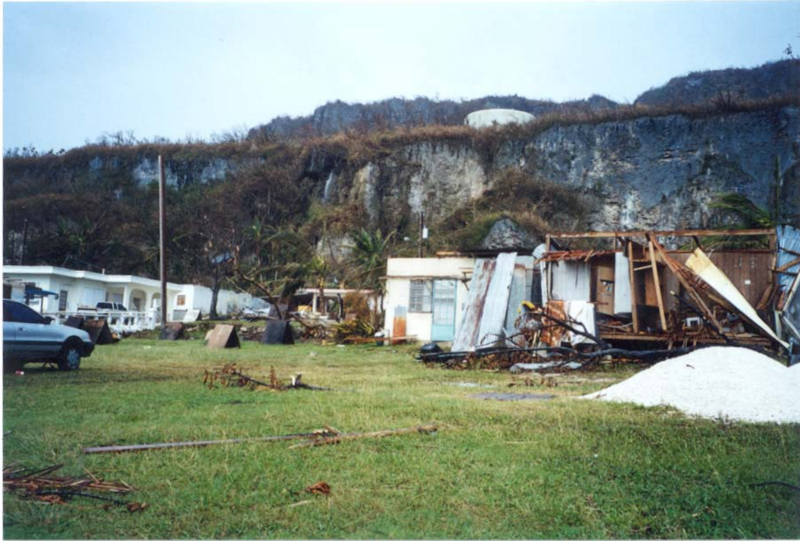
Figure 33. Destroyed wooden house and relatively unscathed reinforced concrete house in eastern Songsong Village, Rota, CNMI.
