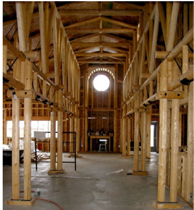
Figure 2. Six-inch-diameter lodgepole pine used in 5,000-ft 2 library under construction in Darby, Montana.
