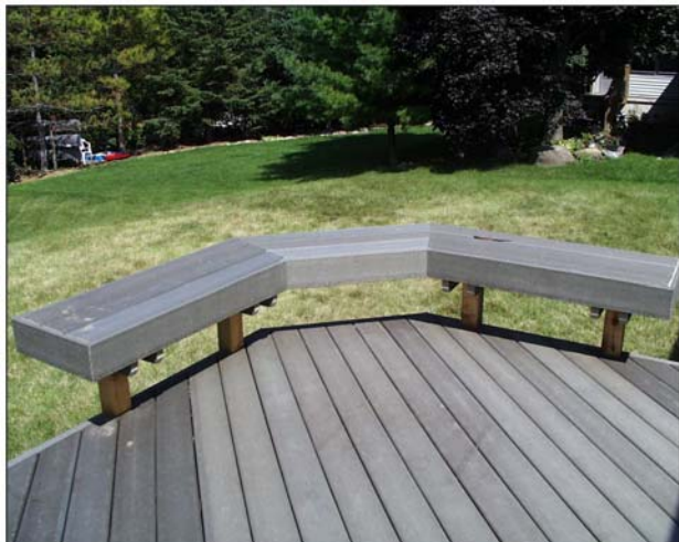
Researchers at the Forest Products Laboratory evaluated how well structures made from wood–plastic composites, such as this deck, hold up to UV exposure and fungal attack.
