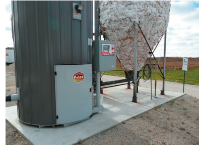
Pelco boiler and fuel hopper
