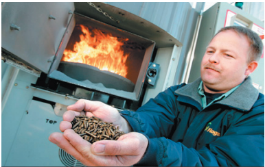
In 2004, Agrecol converted their heating system from LP, and now heats their entire production facilities with native grass pellets
