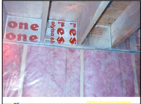
Interior Basement Insulation
