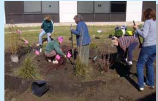
Master Gardeners construct a demonstration rain garden in Gloucester County, New Jersey
