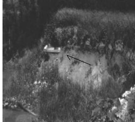
Figure 8. Note location of concrete pad for road culvert relative to current stream location and lack of vegetation in the midbank region.
