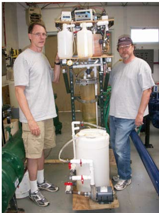
Water Survey researchers Tom Holm and Gary Peyton operate the Fenton filtration arsenic removal unit during pilot tests at the water treatment plant at Monticello, Illinois. The pilot unit is stored on site between experiments for ready availability during optimum treatment conditions. The glass column (bottom of unit) is the flocculation basin and contains a sand filter. Plastic containers (middle level) are the aeration basin and chemical reservoirs, and pumps (top level) supply treatment chemicals.
