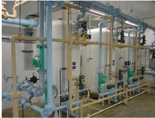
With IWT staff advice on proper treatment, this accelerator at W. Howe Development Center water plant operates past its expected life span.
