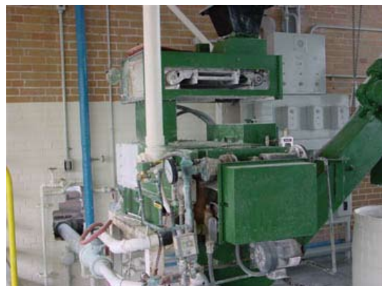
Ion exchange softeners remove hardness salts to prevent deposits from fouling equipment and hot water systems at Dwight Correctional Center.
