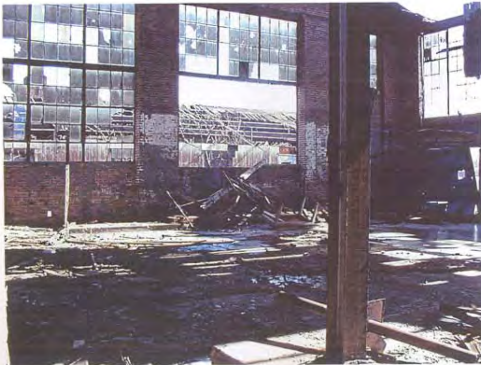
Photograph 2: Example of dilapidated building on the Standard Chlorine site
