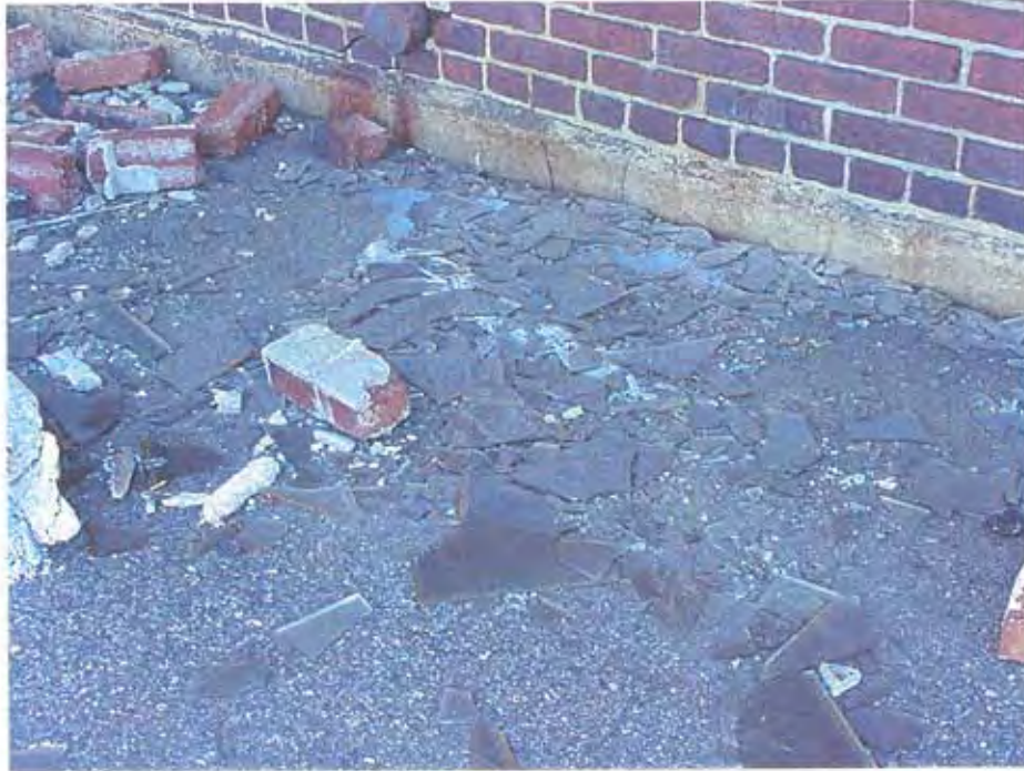
Photograph 1: Broken bricks and glass on the Standard Chlorine site
