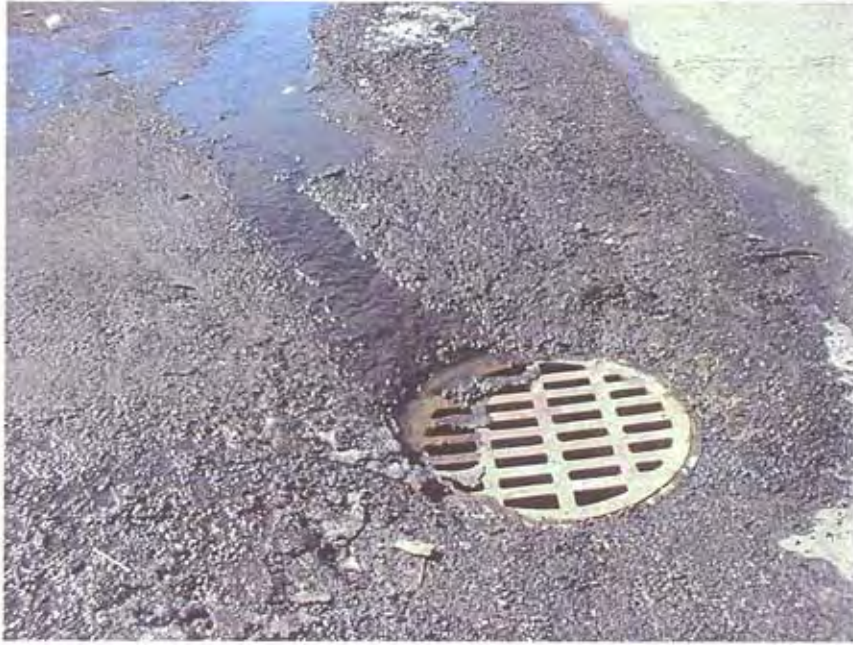
Photograph 13: Storm drain located on the driveway shared between Standard Chlorine and the former Diamond Shamrock site
