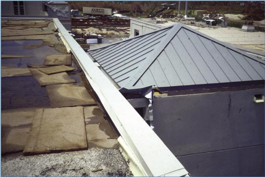
Figure 6-9 The metal roof is over a stair tower. The irregularity created by the stair tower caused turbulence that resulted in wind speed-up.
