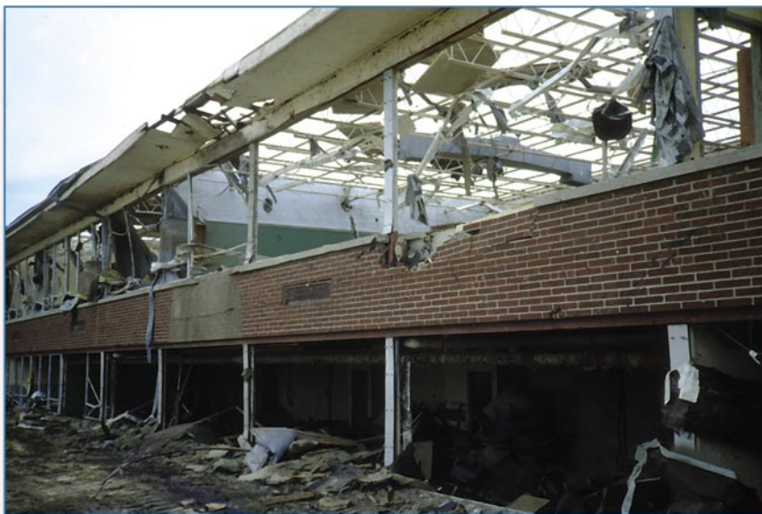
Figure 6-10 This high school in northern Illinois was heavily damaged by a strong tornado.
