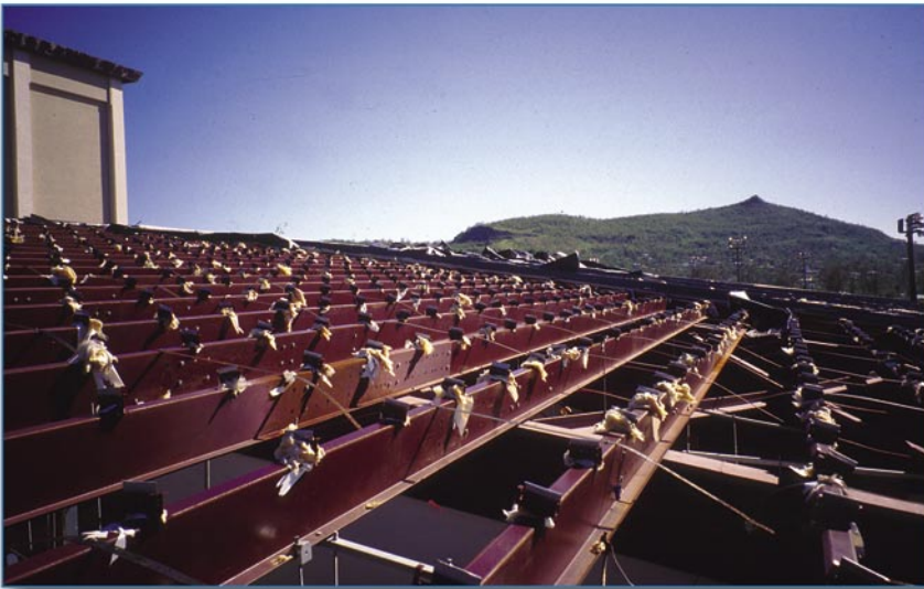
Figure 6-17 This newly-constructed gymnasium had a structural metal roof panel (3-inch trapezoidal ribs at 24 inches on center) applied over metal purlins. The panels detached from their concealed clips. A massive quantity of water entered the school and buckled the wood gym floor.
