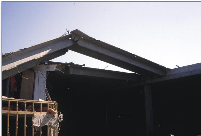
Figure 6-24 Several of the precast twin-Tee roof and wall panels collapsed. The connection between the roof and wall panels provided very little uplift load resistance. This roof panel lifted because of combined effects of wind uplift and pretension.
