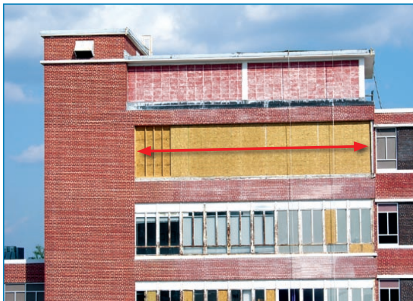
Figure 3-110: Wind pressure caused the window frames on the upper floor to fail (red arrow). Hurricane Katrina (Mississippi, 2005)
