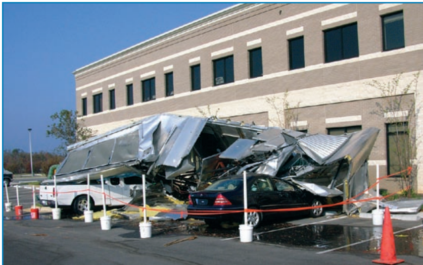
Figure 3-69: Although this 18,000-pound HVAC unit was attached to its curb with 16 straps, it blew off during Hurricane Ivan. (Florida, 2004)
