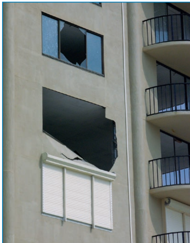
Figure 3-113: The lower window assembly was protected with a motorized shutter. Hurricane Ivan (Florida, 2004)
