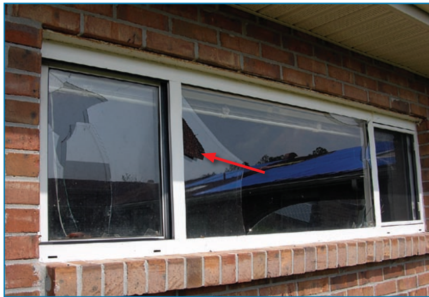
Figure 3-85: A small piece of asphalt shingle (red arrow) broke the window at this nursing home. Hurricane Katrina (Mississippi, 2005)
