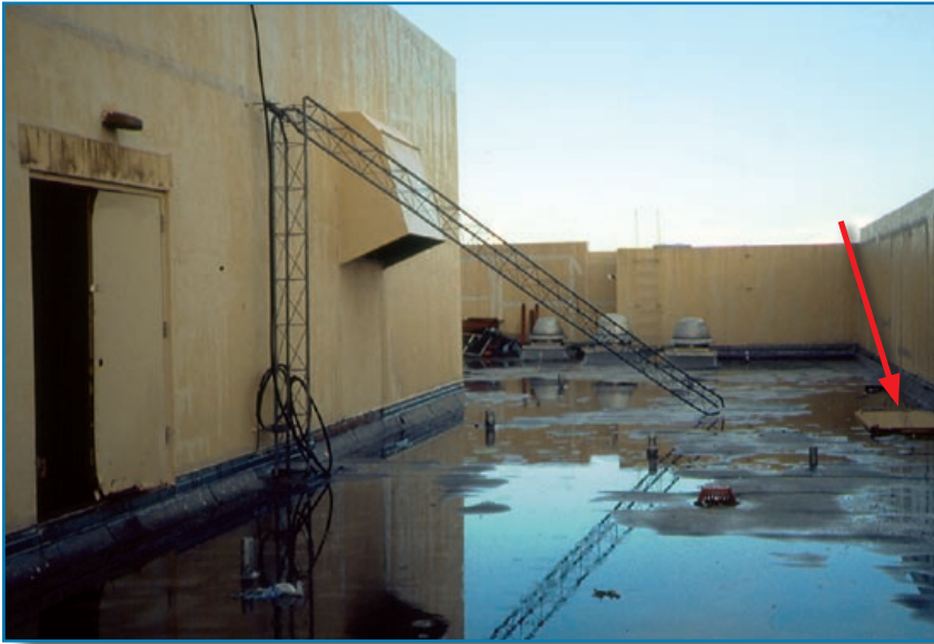
Figure 3-118: The antenna at this hospital collapsed and was whipped back and forth across the roof membrane. Hurricane Andrew (Florida, 1992)
