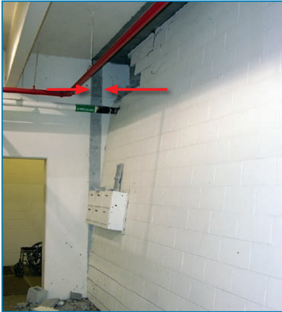
Figure 3-44: The red arrows show the original location of a CMU wall that nearly collapsed following a rolling door failure. Hurricane Charley (Florida, 2004)
