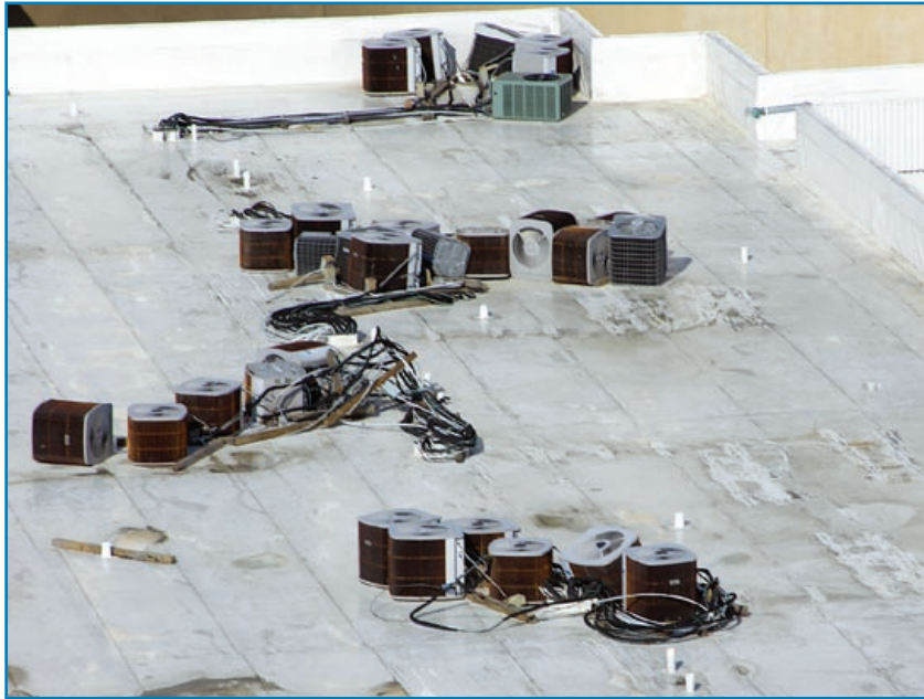
Figure 3-73: Sleeper-mounted condensers displaced by high winds. Hurricane Katrina (Mississippi, 2005)
