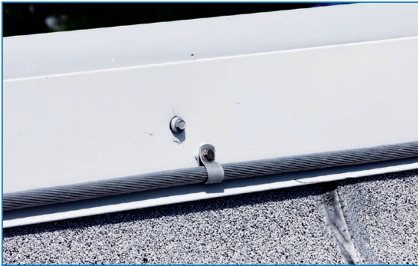
Figure 3-97: This conductor was attached to the coping with a looped connector. Hurricane Katrina (Mississippi, 2005)
