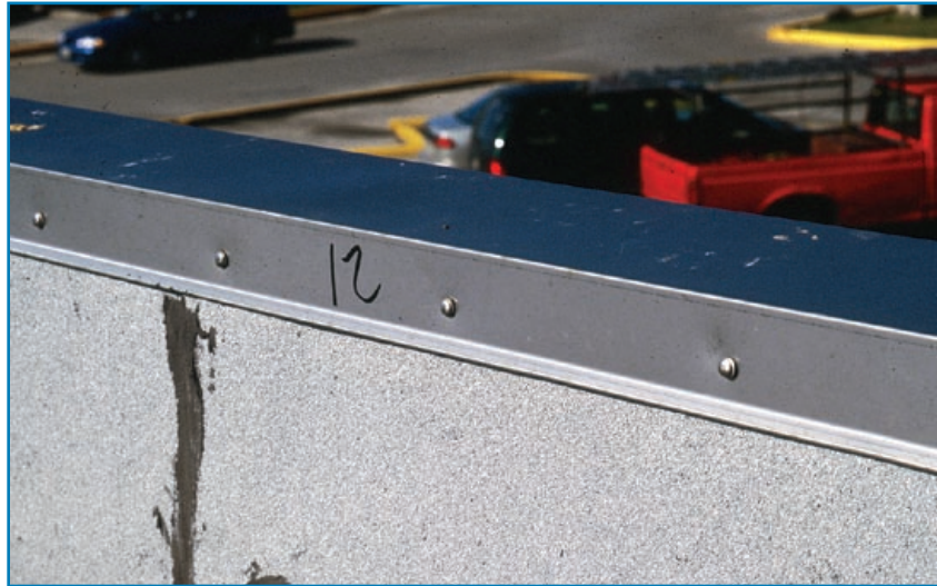
Figure 3-63: Both vertical faces of the coping were attached with exposed fasteners instead of concealed cleats. Typhoon Paka (Guam, 1997)
