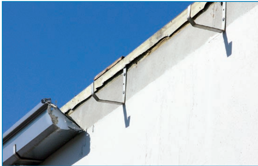
Figure 3-64: This gutter, supported by a type of bracket that provides no significant uplift resistance, failed when wind lifted it together with the metal edge flashing that lapped into the gutter. Hurricane Francis (Florida, 2004)
