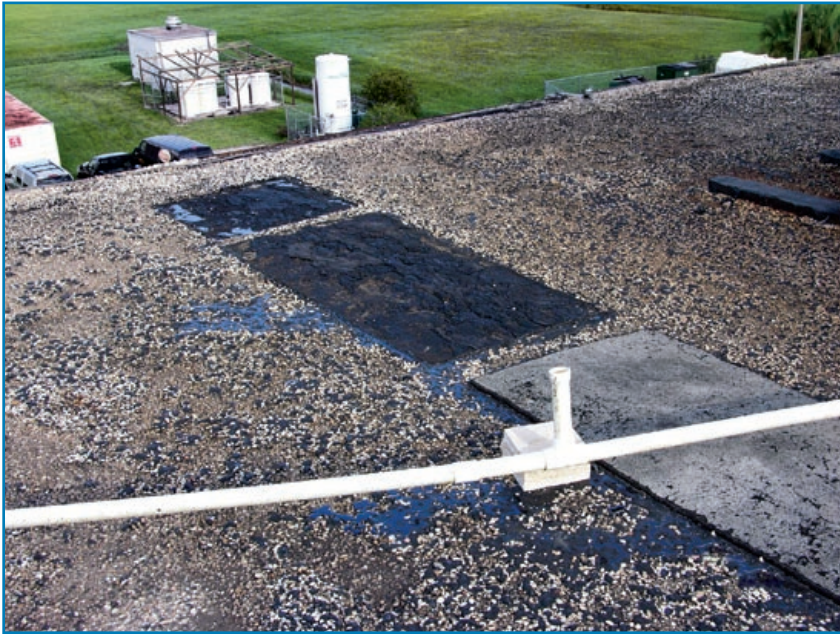
Figure 3-92: To avoid walkway pad blow off, as occurred on this hospital roof, walkway pads are not recommended. Hurricane Charley (Florida, 2004)
