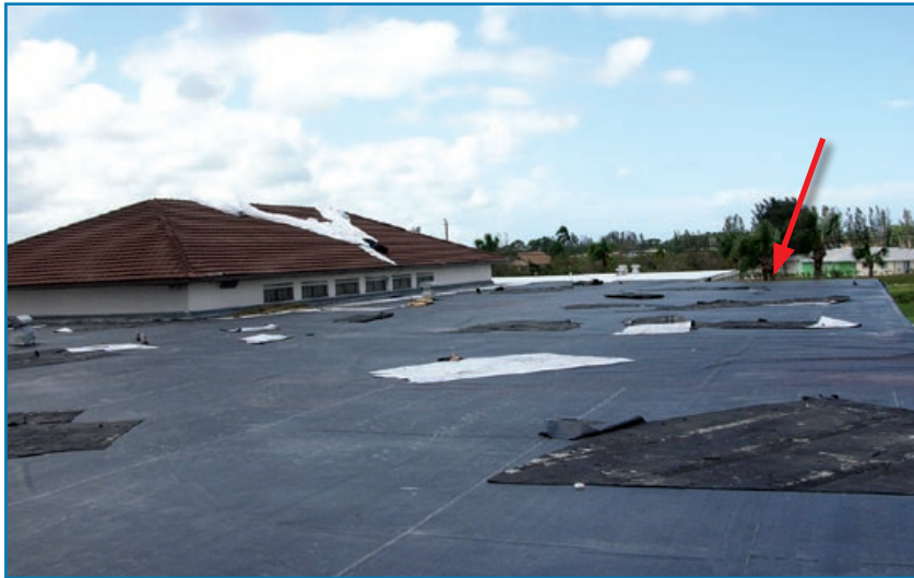
Figure 3-65: The original modified bitumen membrane was blown away after the gutter lifted in the area shown by the red arrow (the black membrane is a temporary roof). Hurricane Francis (Florida, 2004)
