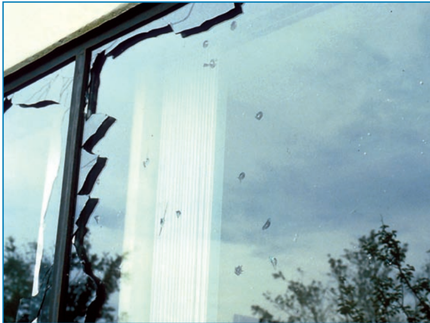
Figure 3-13: The outer window panes were broken by aggregate from a built-up roof. Hurricane Hugo (South Carolina, 1989)
