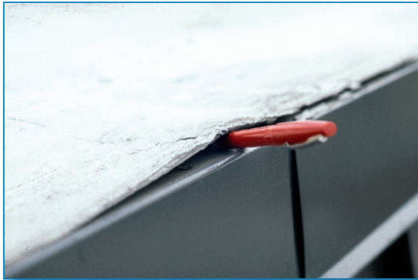
Figure 3-61: The ink pen shows an opening that the wind can catch, and cause lifting and peeling of the membrane.
