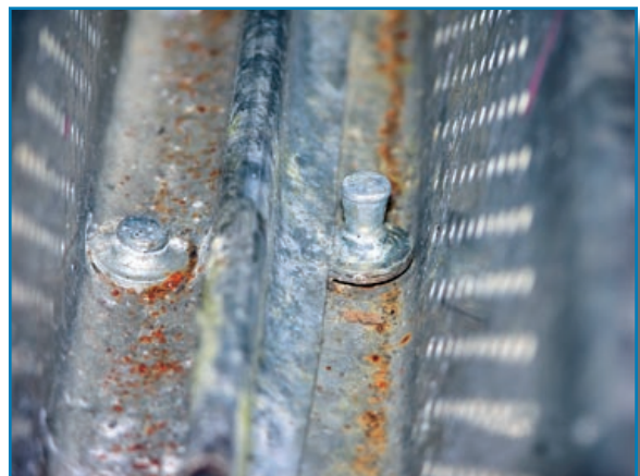
Figure 3-25: View looking along a sidelap of a deck attached with powder-driven pins. The right pin does not provide adequate uplift and shear resistance.
