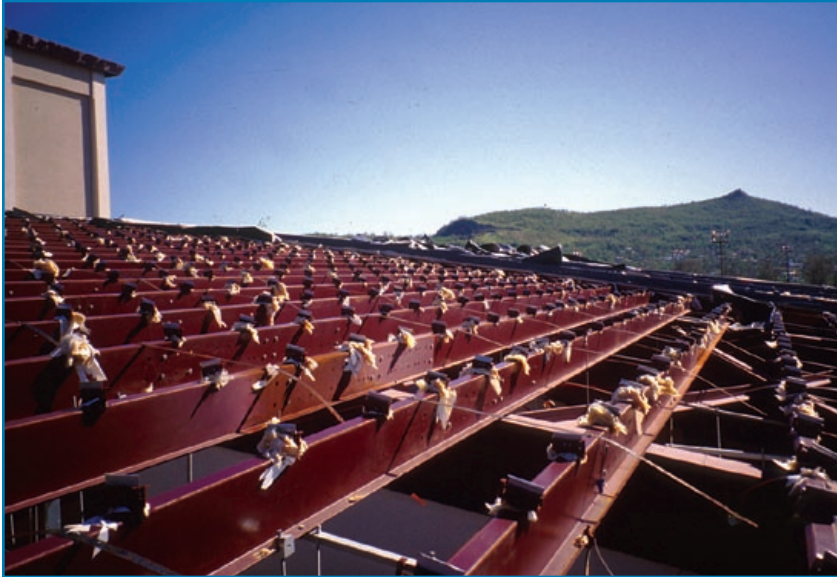
Figure 3-17: A massive quantity of water entered the building after the roof blew off. Typhoon Paka (Guam, 1997)
