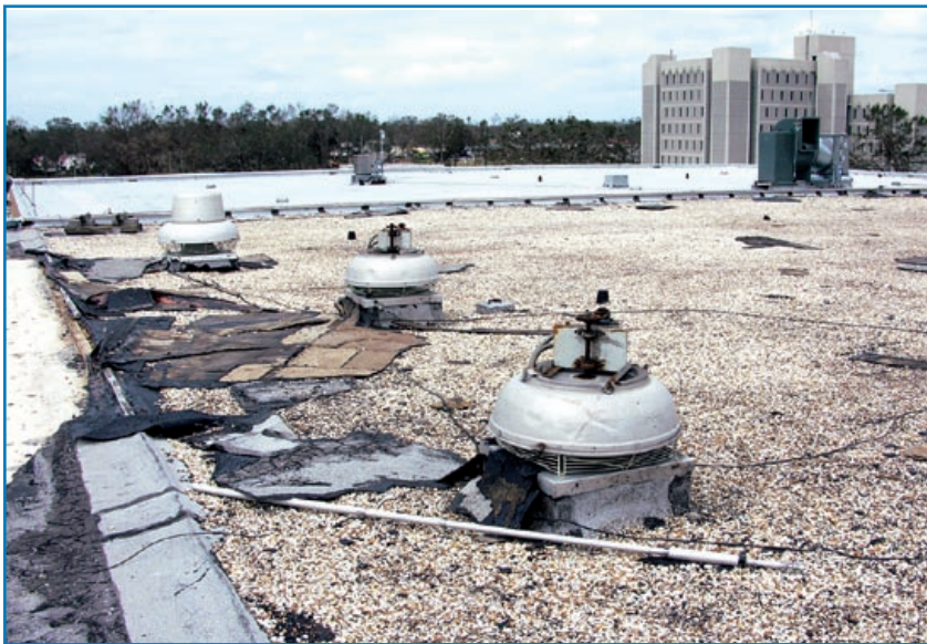
Figure 3-70: Cowlings blew off two of the fans on a police building that housed the county's EOC. Hurricane Ivan (Florida, 2004)
