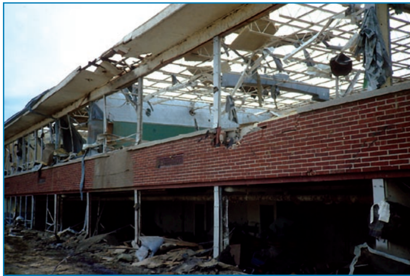
Figure 3-102: A Northern Illinois school heavily damaged by a strong tornado in 1990
