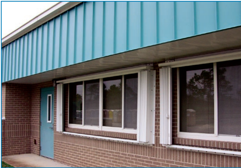
Figure 3-111: This school has accordion shutters. Hurricane Ivan (Florida, 2004)
