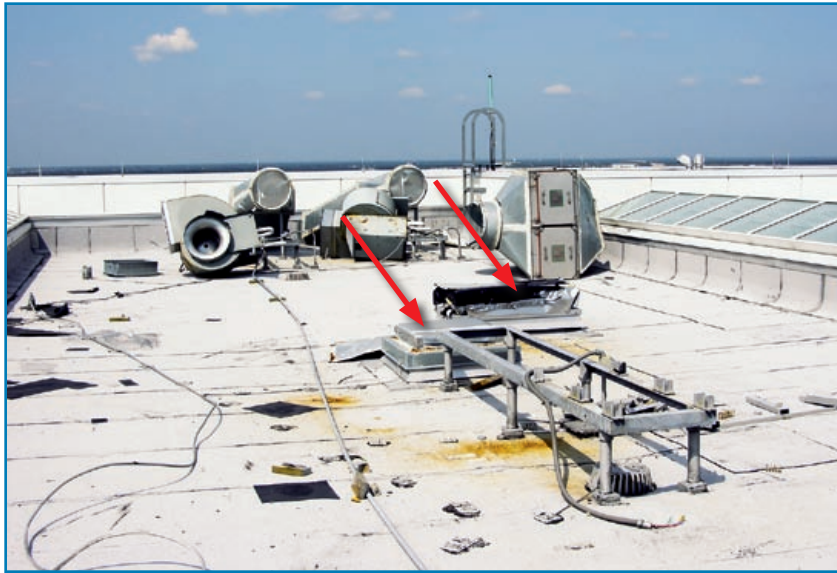
Figure 3-20: Temporary coverings placed over two large openings in the roof that were left after the ductwork blew away. Hurricane Katrina (Mississippi, 2005)
