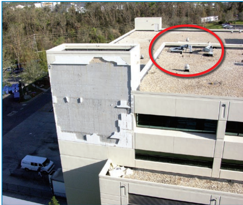
Figure 3-55: EIFS blown off a cast-in- place concrete wall. Note the damaged rooftop ductwork. Hurricane Ivan (Florida, 2004)
