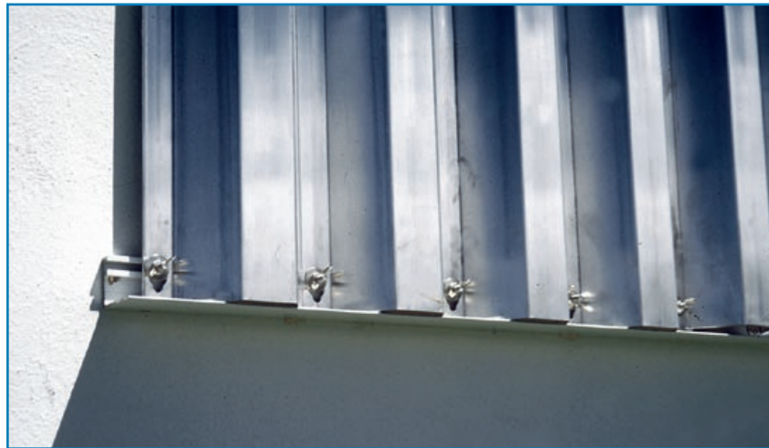
Figure 3-112: Illustrates a metal panel shutter. Hurricane Georges (Puerto Rico, 1998)
