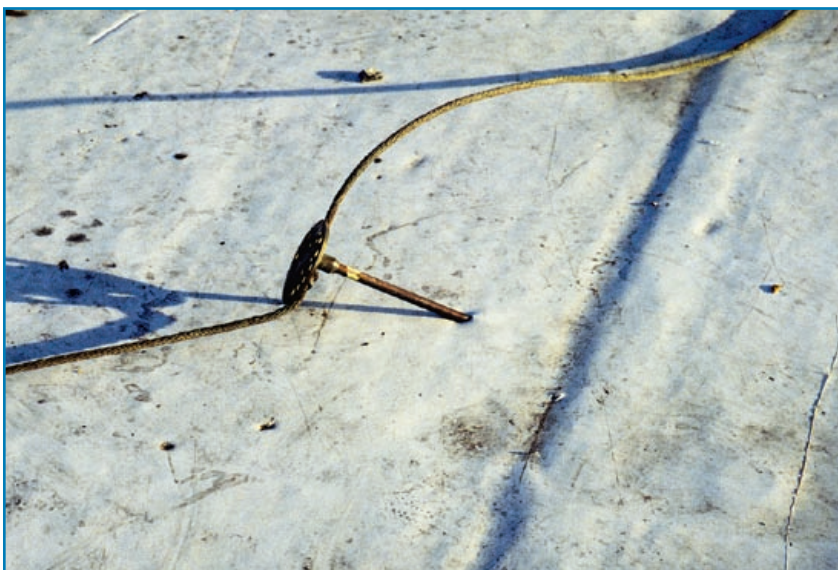
Figure 3-94: A displaced air terminal that punctured the membrane in several locations. Hurricane Marilyn (U.S. Virgin Islands, 1995)
