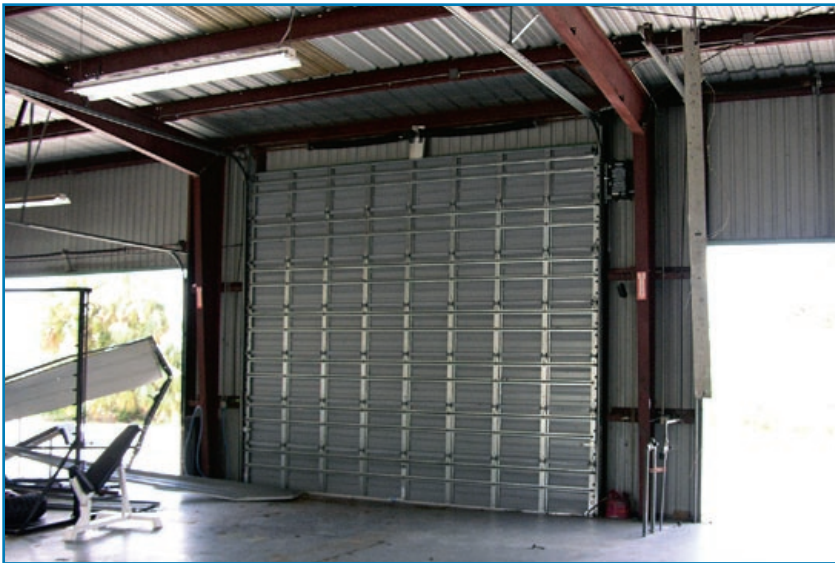
Figure 3-109: The new door in the center performed very well, but the older doors on either side of it were blown away. Hurricane Charley (Florida, 2004)
