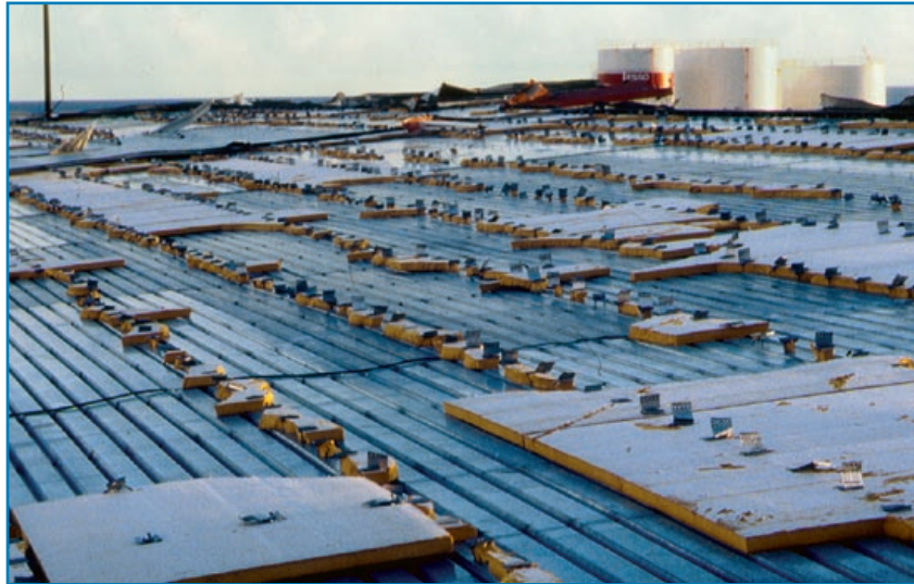
Figure 3-87: Significant interior water damage and facility interruption occurred after the standing seam roof blew off. Hurricane Marilyn (U.S. Virgin Islands, 1995)
