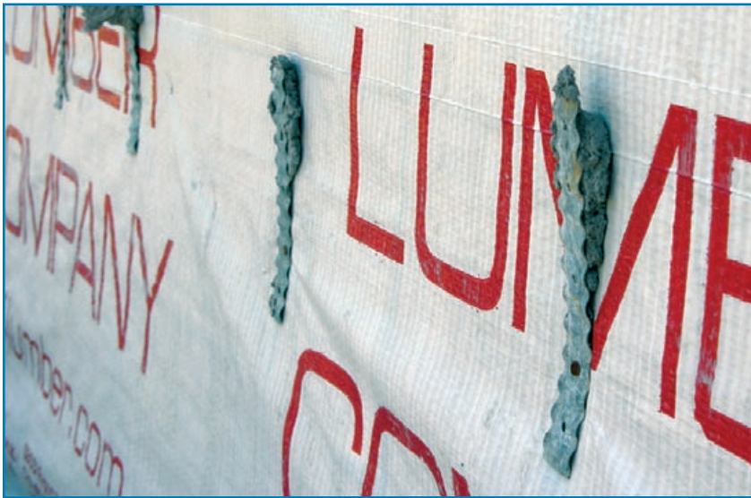
Figure 3-47: These four ties were never embedded into the mortar joint.
