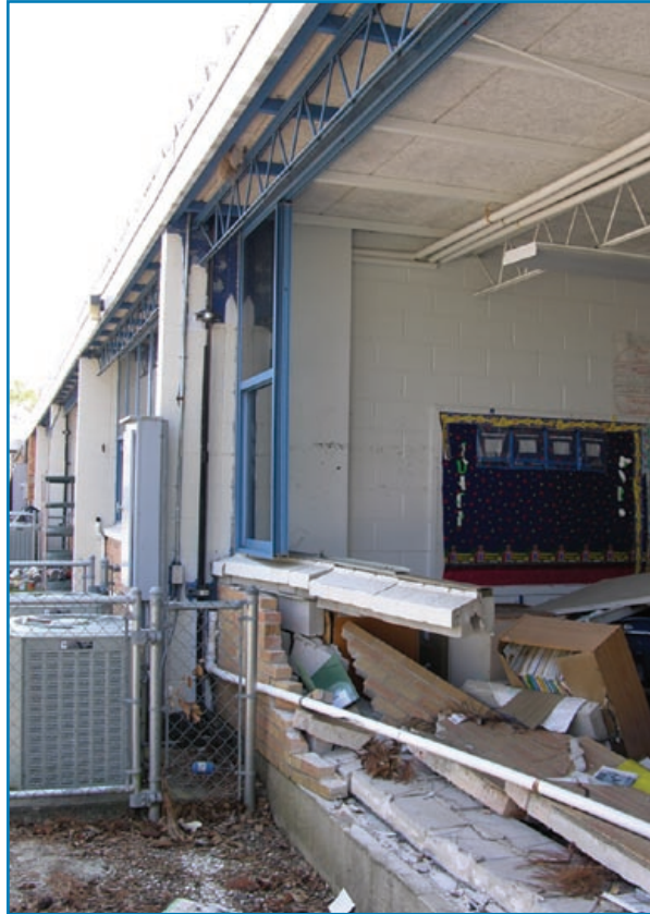
Figure 3-105: Several walls at this school collapsed. Windows were located above a non- load-bearing masonry wall. Hurricane Katrina (Mississippi, 2005)
