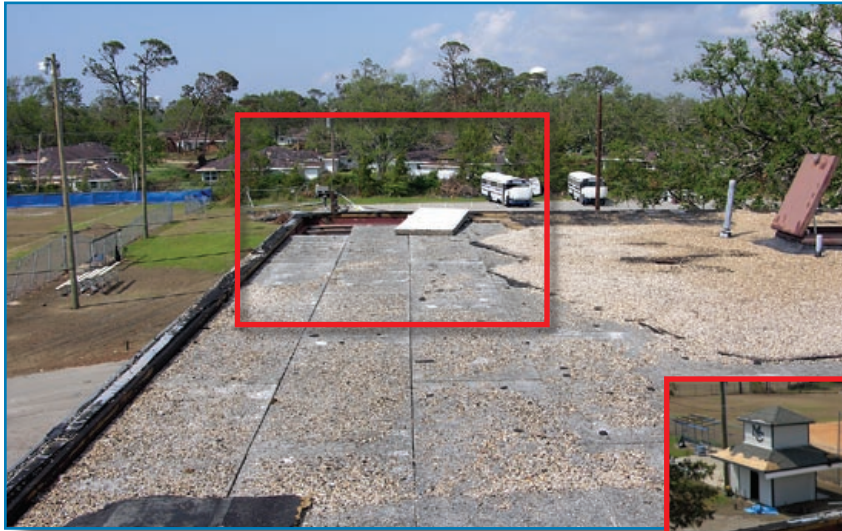
Figure 3-106: The school's built-up roof blew off after one of the cementitious wood-fiber deck panels detached from the joists. Hurricane Katrina (Mississippi, 2005)
