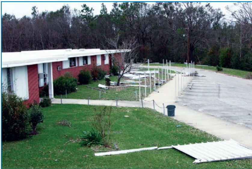
Figure 3-28: The destroyed walkway canopy in front of a school became wind-borne debris. Hurricane Ivan (Florida, 2004)
