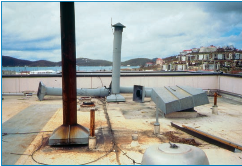
Figure 3-76: Three of the five stacks that did not have guy-wires were blown down. Hurricane Marilyn (U.S. Virgin Islands, 1995)
