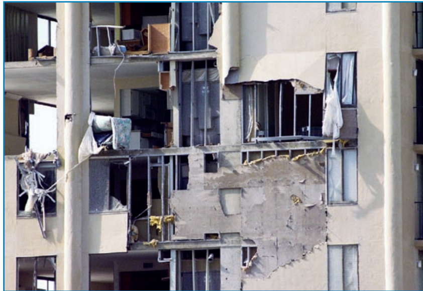
Figure 3-57: The stucco wall failure was caused by inadequate attachment between the stud tracks and the building's structure. Hurricane Ivan (Florida, 2004)
