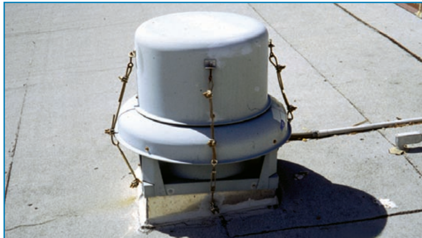
Figure 3-71: Cables were attached to prevent the cowling from blowing off. Typhoon Paka (Guam, 1997)
