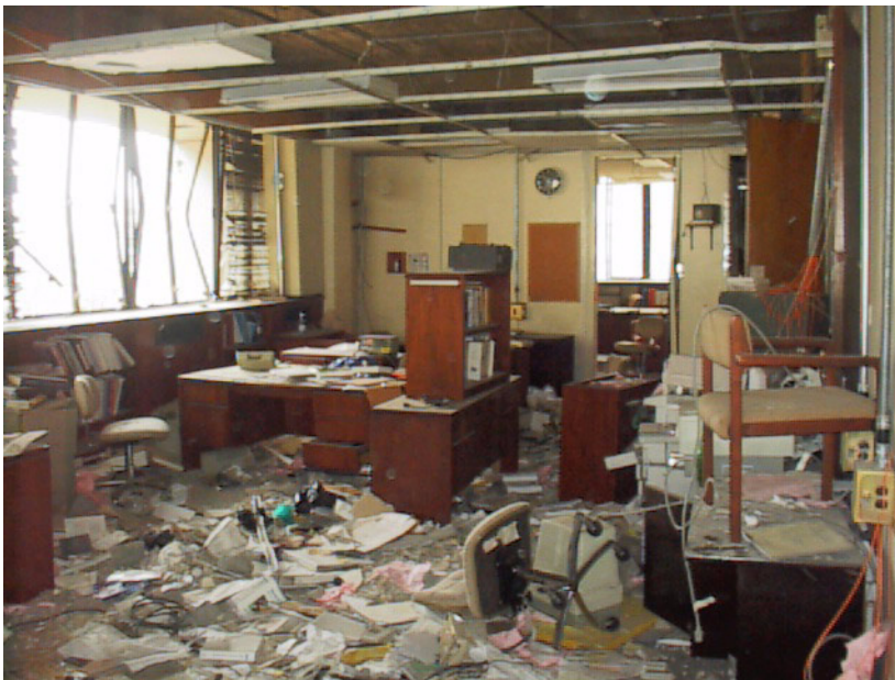
Figure 4-5 Photograph showing non-structural damage in building impacted by blast
