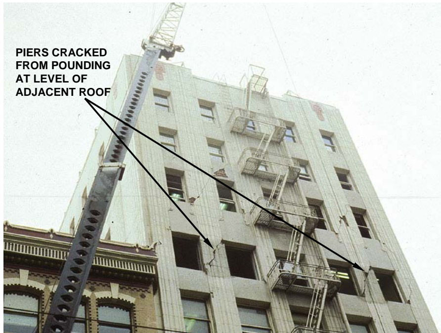
Figure 3-12 Photo showing damage caused by the pounding of a 10-story steel-frame building (with masonry infill walls) against a seven-story building. Most of the cracking damage to the piers of the taller building was at the roof line of the shorter building (Most of the cracking damage to the piers of the taller building was at the roof line of the shorter building. ATC-20 Training Slide Set photo)
