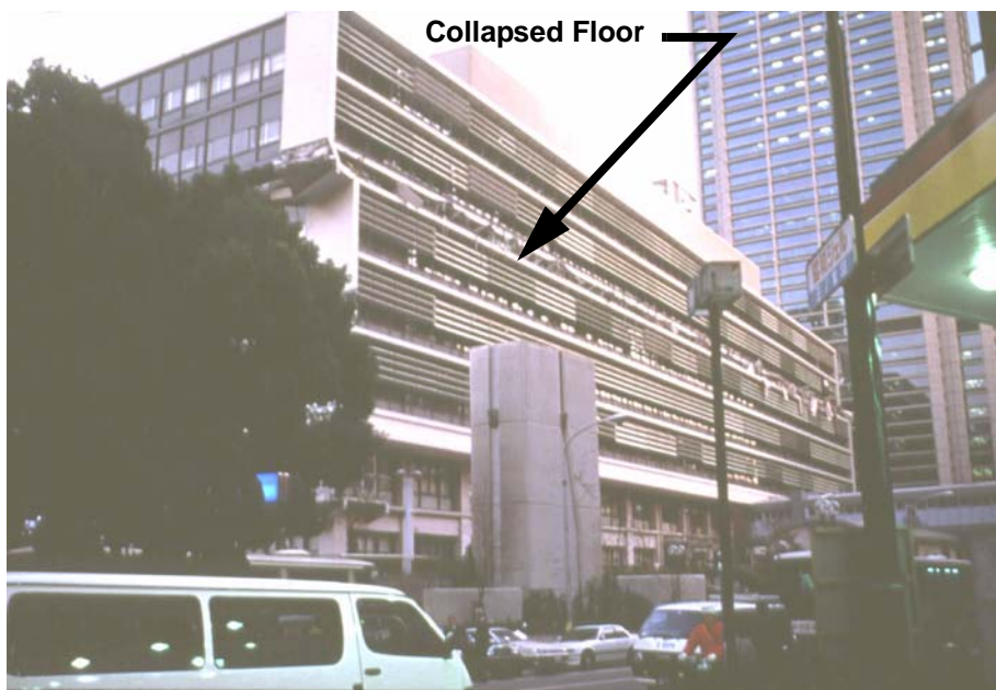
Figure 3-2 Eight-story reinforced-concrete-frame office building in Kobe, Japan that partially collapsed during the magnitude-7.8 earthquake of January 17, 1995. Note that the sixth floor is missing, due to collapsed columns at that level. Seismic codes in Japan are essentially equivalent to those in the United States. (photo courtesy of C. Rojahn)
