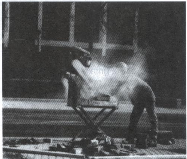
Construction worker sawing masonry without dust control or a respirator.
