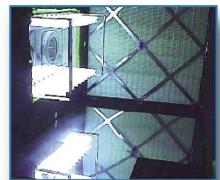
Figure 5-10 UVGI array used for air disinfection with reflective surfaces
