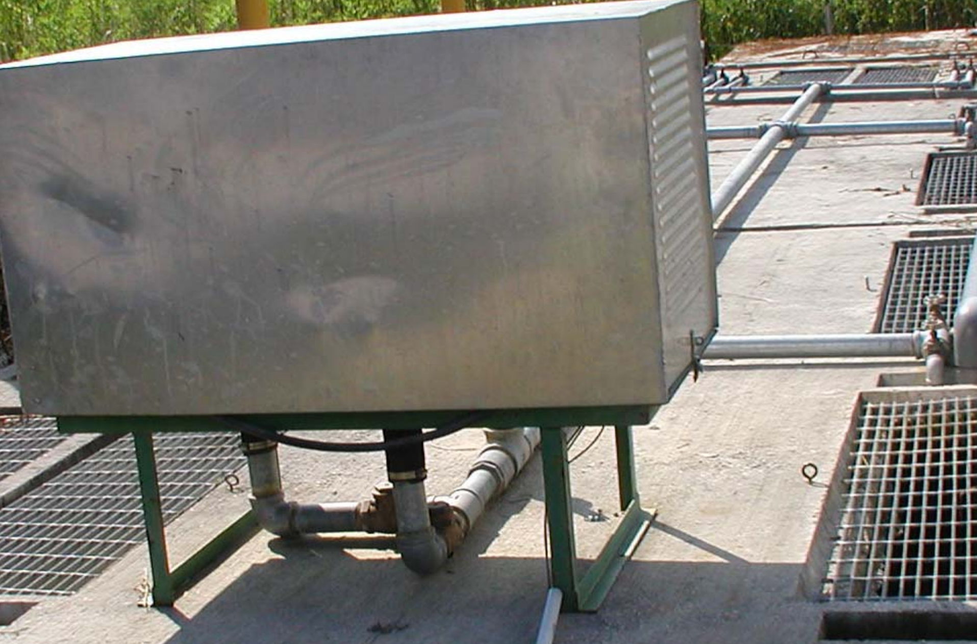
Modular Wastewater Treatment Plants
