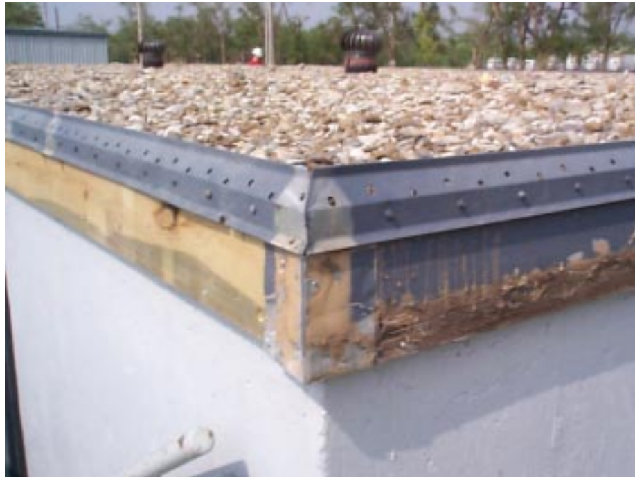
FIGURE 6-15: Ballast roof covering on a community shelter in Wichita, Kansas was a potential source of deadly windborne missiles to those seeking to access the shelter.
