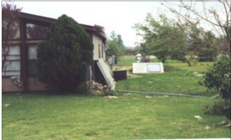
FIGURE 6-4: This precast concrete storm cellar was located immediately behind a residence in Sedgwick County, Kansas. This residence and shelter were on the periphery of a violent tornado path.
