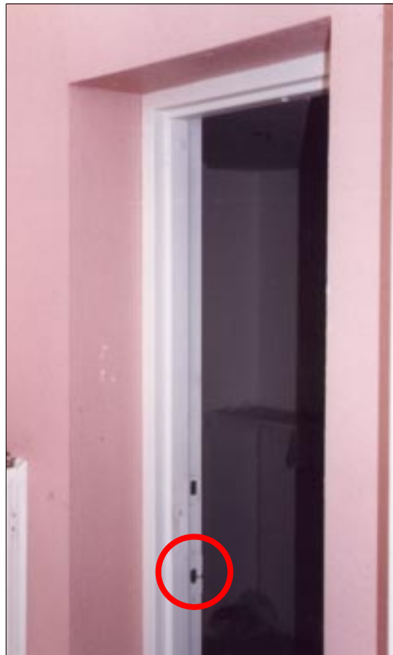
FIGURE 6-14: Shelter door of home in Del City, Oklahoma, showing an insufficient deadbolt locking device. The circled area on the door frame is the catch for the only latching mechanism on the door.
