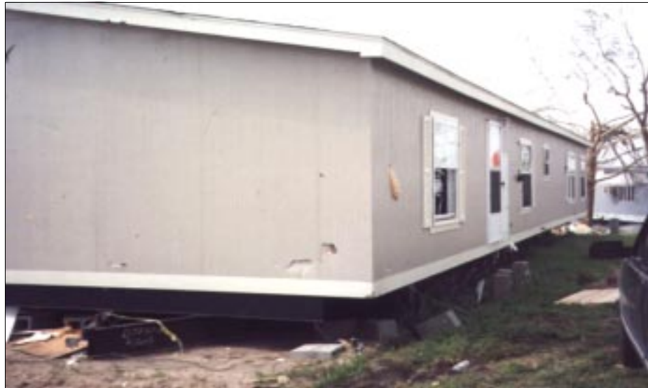
FIGURE 4-61: Manufactured home laterally shifted from wind force generated along the periphery of a violent tornado, Wichita, Kansas.
