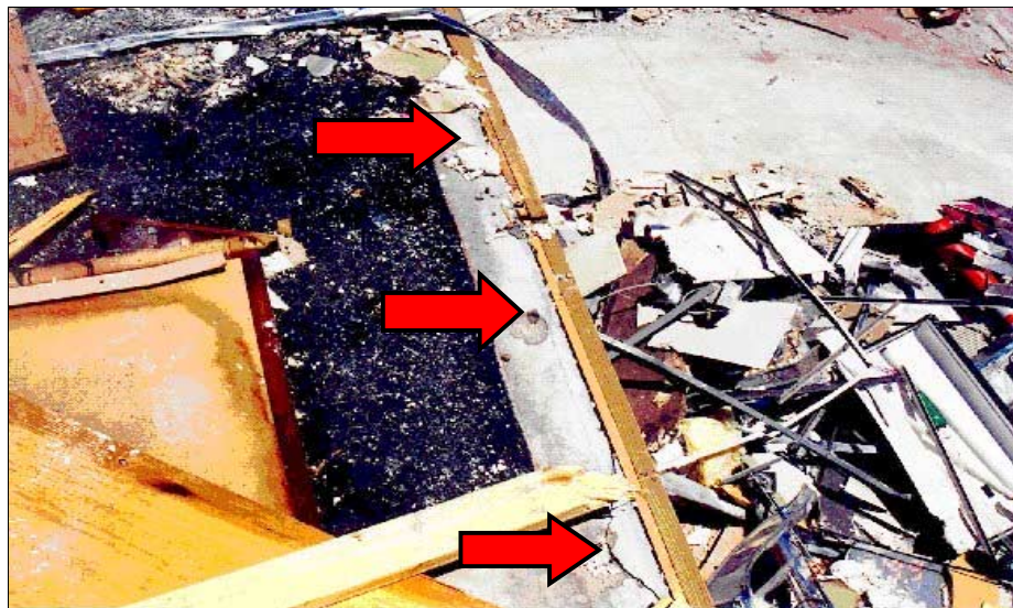
FIGURE 5-22: Attachments of lower plates for wall to hollow core plank using power driven anchors failed when required to carry loads generated by the winds of a moderate tornado vortex. This motel was located in Midwest City, Oklahoma.
