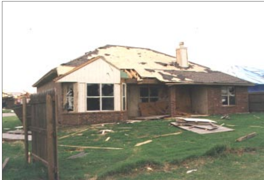
FIGURE 4-26: Damage to back of home in the Country Place Subdivision in Oklahoma City, was limited to several window failures and minor roof damage. The home was located along the periphery of a violent tornado.
