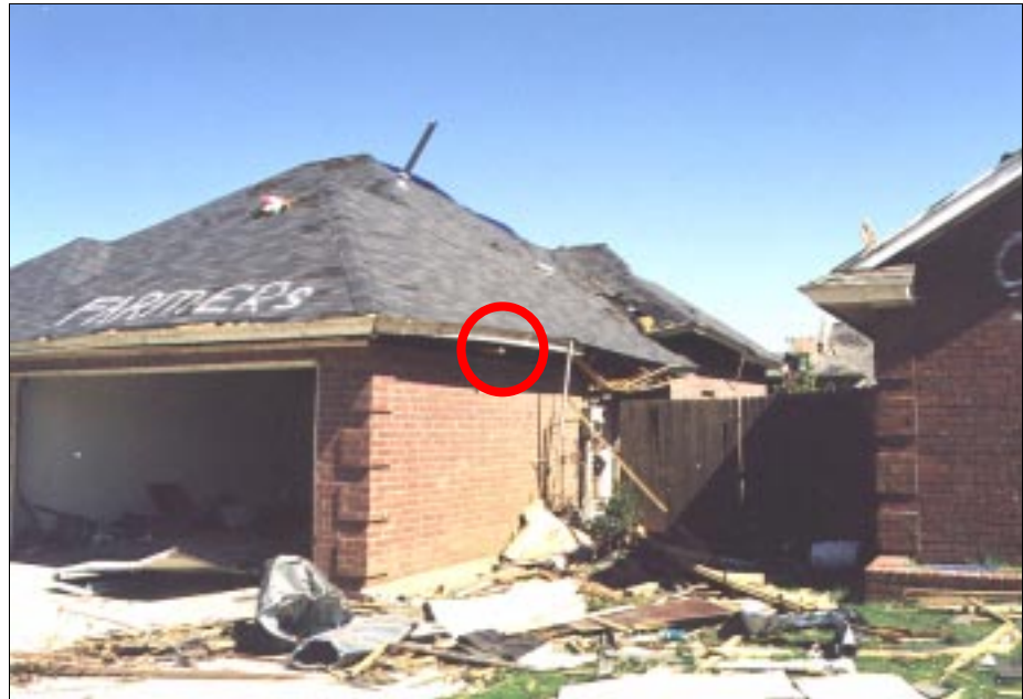
FIGURE 4-21: A 2x4 member extends out of the gap that runs the length of this garage wall between the top of the wall and the roof framing
