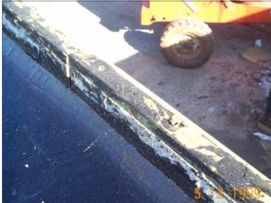
Figure 5.23: Nailer at the roof of the hospital in Stroud, Oklahoma. The roof surface in this photo was replaced prior to this photo, but the same nailer was used again.
