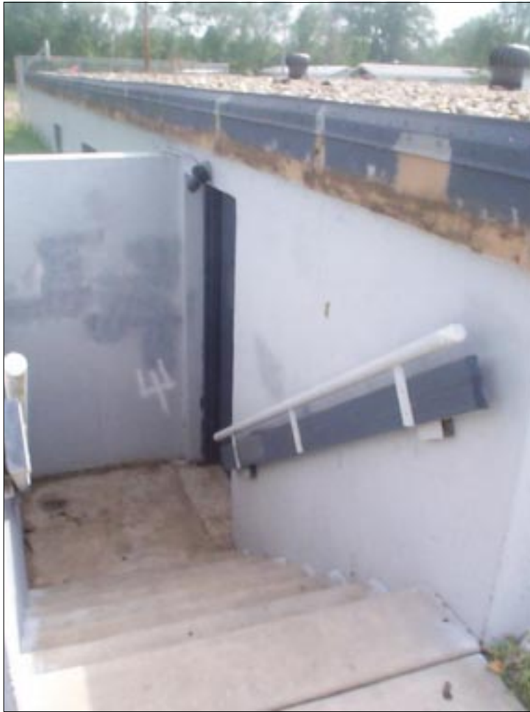
FIGURE 6-16: Stairway leading to entrance of manufactured home community shelter, Wichita, Kansas. The only means of accessing this structure were this stairway and an identical one at the other side of the shelter.
