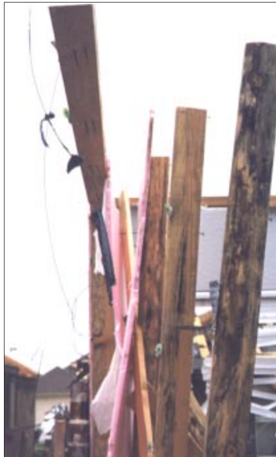
FIGURE 4-9: Failures of the connection of the double-top-plate to the supporting studs below by home located in Moore, Oklahoma. This home was located along the periphery of a violent tornado.
