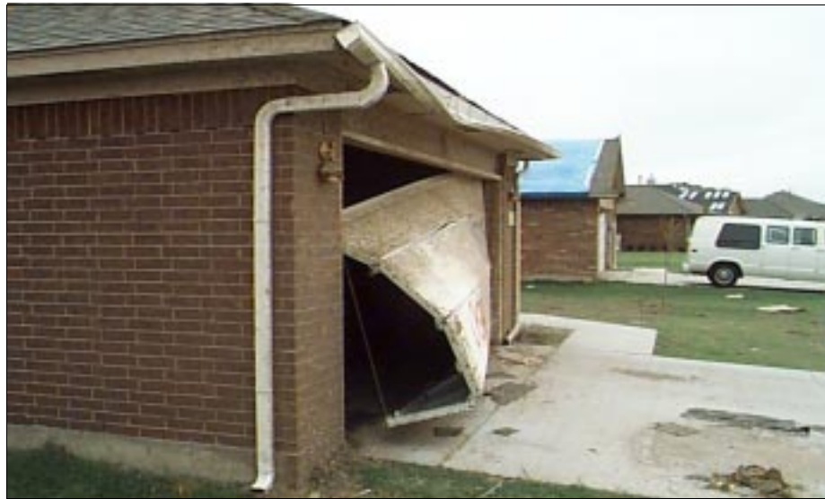
FIGURE 4-18: This double-width garage door failed under a suction load in Moore, Oklahoma.
