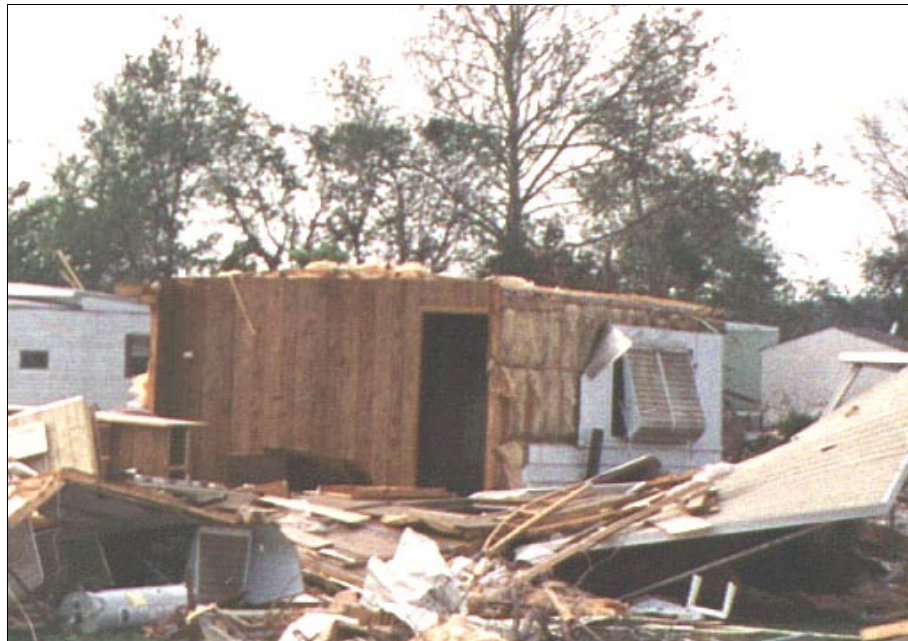
Figure 4-54: Roof and wall damage experienced due to inadequate resistance to lateral and uplift wind forces associated with straight inflow winds of a moderate tornado, Wichita, Kansas.
