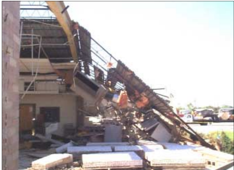
FIGURE 5-13: Collapsed roof structure and exterior at Kelly Elementary School in Moore, Oklahoma struck by the vortex of a violent tornado.
