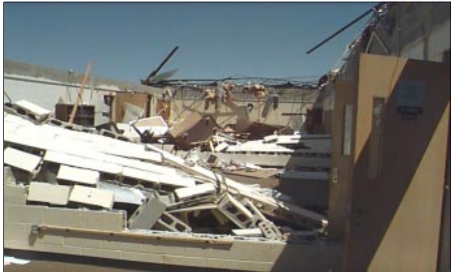
FIGURE 6-35: The non-reinforced interior CMU walls in this area of Kelly Elementary collapsed after the roof system was removed by vortex winds of a violent tornado.
