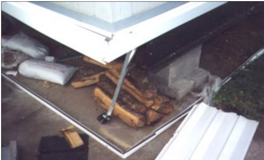
FIGURE 4-59: View of anchor strap and attachment indicating lateral shifting of a manufactured home, Haysville, Kansas. This home was located along the periphery of a violent tornado.
