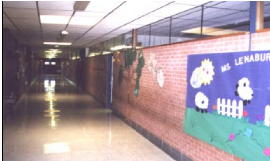
FIGURE 6-31: Northmoor Elementary place of refuge, Moore, Oklahoma - double loaded corridor with clerestory windows. This corridor offers little protection from a violent tornado as shown in a school of similar design in Figure 6-32.
