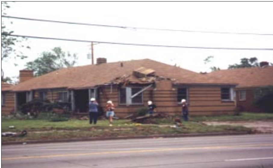
FIGURE 4-46: Chimney failure onto roof of single family attached housing, Wichita, Kansas. This building was located along the periphery of a severe tornado.
