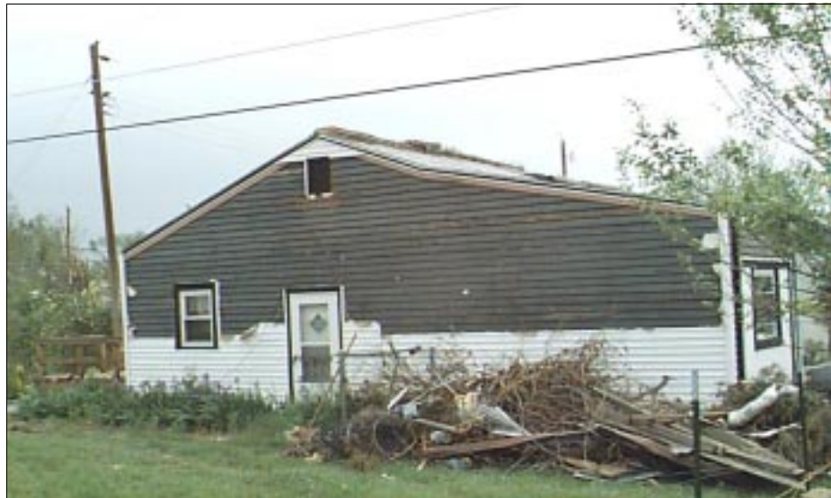
FIGURE 4-16: The vinyl (white) that was installed over wood siding experienced damage; however, the wood siding was undamaged. The home was located along the periphery of a violent tornado in Wichita, Kansas.
