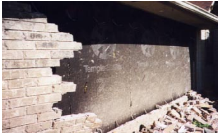
FIGURE 4-32: Failure of masonry veneer wall of a home located along the periphery of a violent tornado, Moore, Oklahoma.
