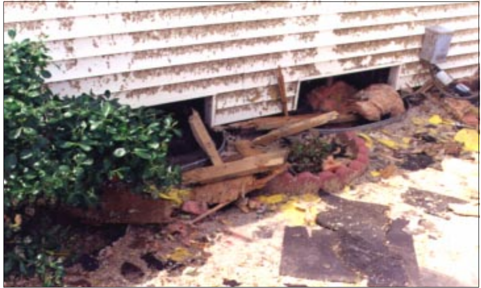
FIGURE 6-19: Basement windows of residential home, showing vulnerability to debris.
