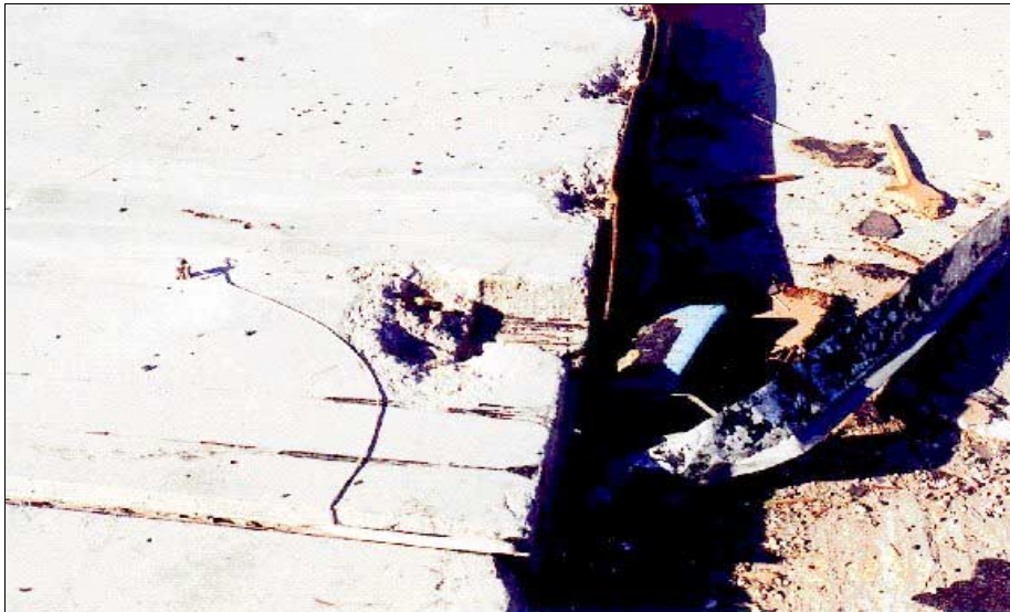
FIGURE 5-17: Top of failed tilt-up wall.
