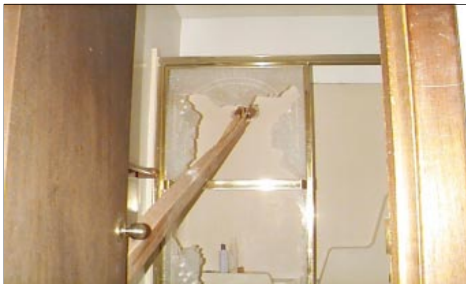
FIGURE 6-24: A 10-ft long 2-in by 6-in missile penetrated the exterior wall of this house in Wichita, Kansas, which was sheathed with hardboard panels. The missile, which was generated from the vortex of a severe tornado, then penetrated the gypsum board and tile tub enclosure, the tempered glass shower door, and the interior partition near the door frame. At the interior partition, it pierced through a wall stud and projected a few inches into the hallway (Figure 6-25).
