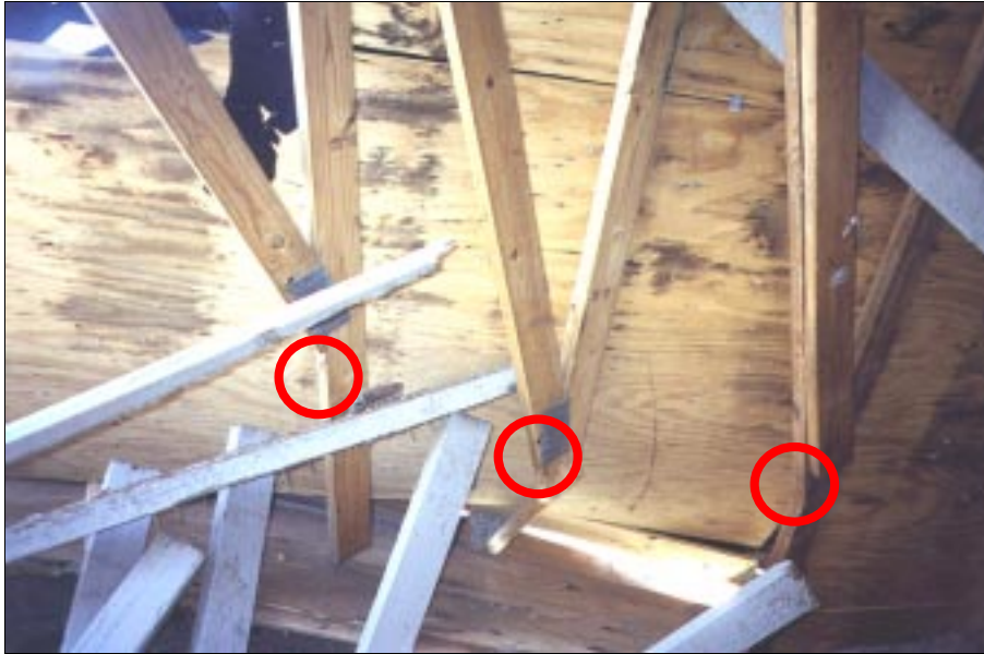
FIGURE 4-7: Roof truss failure. A single nail (circled) was used to connect each truss to the top plate. This house was in Midwest City, Oklahoma and experienced inflow winds from a violent tornado.
