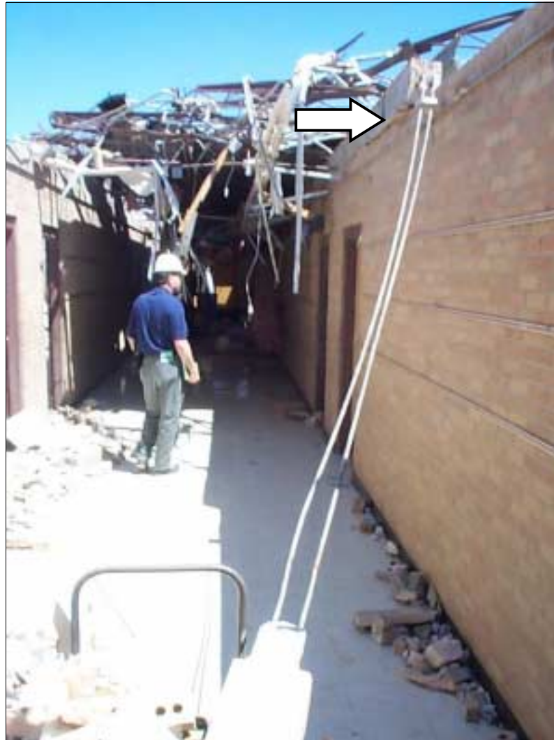
FIGURE 5-3: Kelly Elementary School, in Moore, Oklahoma, hit by vortex of violent tornado. Damage to school displaying separation between the bond beam and supporting wall and separation between bond beam and roof bar joists.
