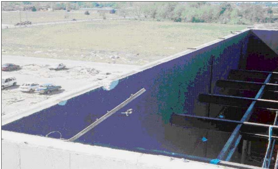
FIGURE 5-14: Roof blown off over top of auditorium at Westmoore High School, Moore, Oklahoma hit by inflow winds of violent tornado.
