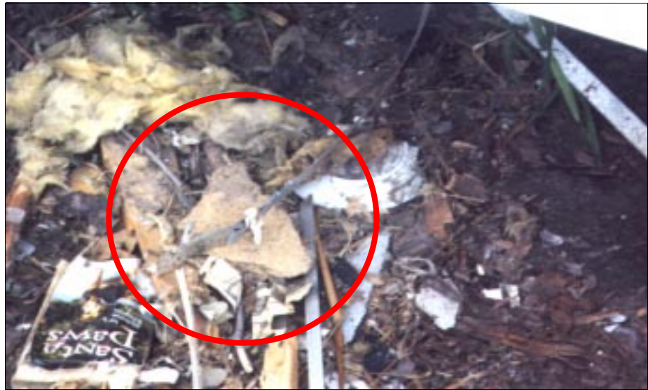
Figure 4-53: Strap torn off from chassis of manufactured home. This home in Wichita, Kansas, was located within the inflow area of a severe tornado.
