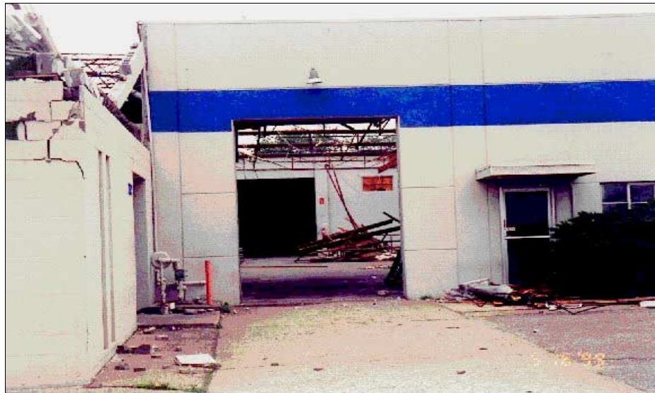
FIGURE 5-19: The tilt-up precast concrete walls in this building did not fail when the roof system failed. Note: many roof joists are still in place. Building was located in Wichita, KS and was hit by moderate tornado vortex.
