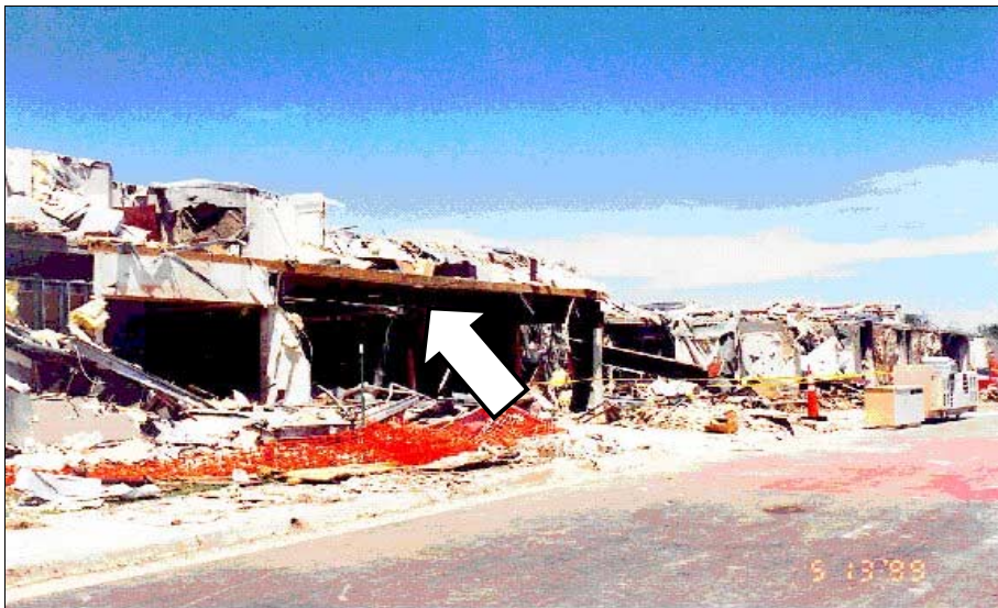
FIGURE 5-11: Motel in Mid West City, Oklahoma that experienced major damage when struck by the vortex of a violent tornado.
