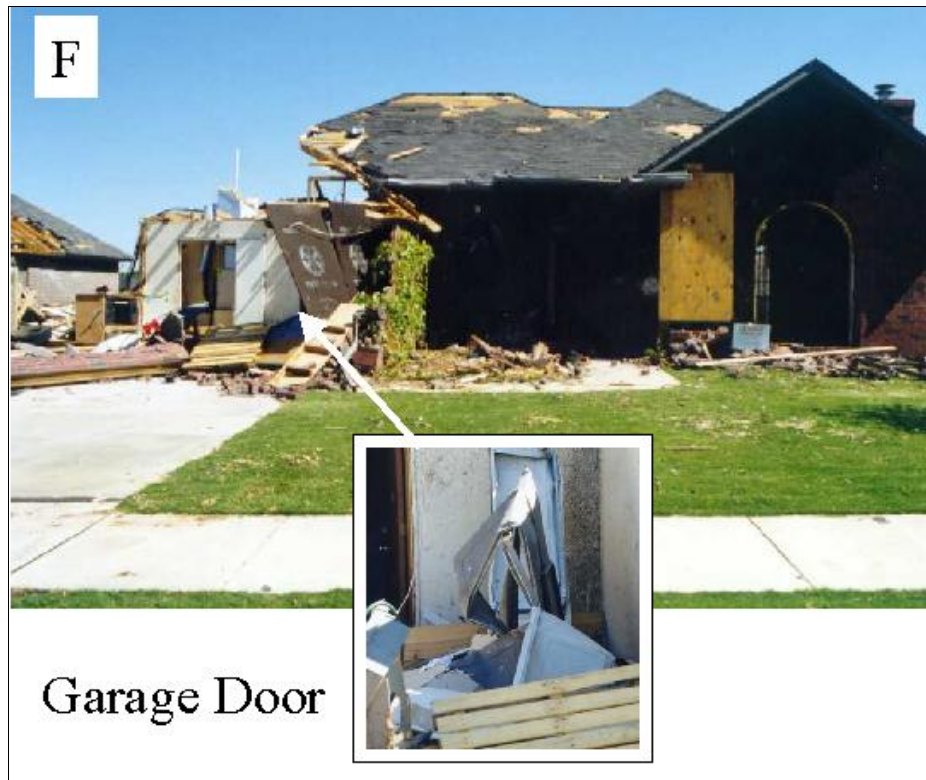
FIGURE 4-22: Garage door failure possibly resulting in the localized partial roof failure on the left side of this home located in Moore, Oklahoma.
