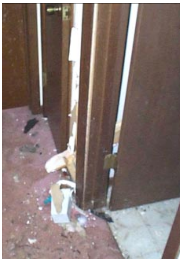
FIGURE 6-25: The missile in Figure 6-24 impacted and broke a 2-in by 4-in wall stud after traveling through the bathroom.
