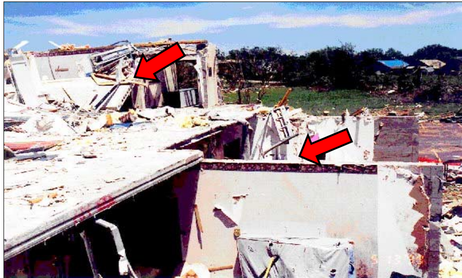
FIGURE 5-21: Hollow-core plank formed on second floor of a Midwest City, Oklahoma, hotel that was struck by the vortex of a moderate tornado.
