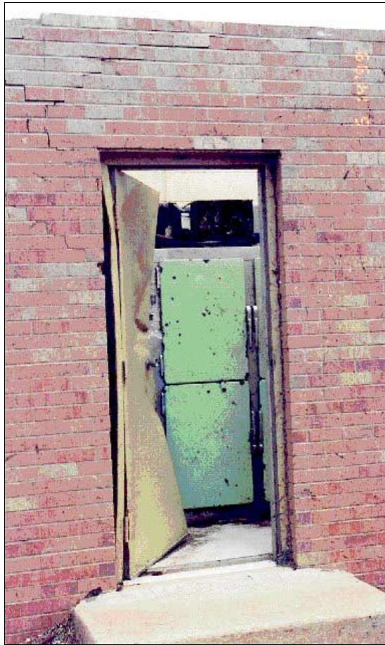
FIGURE 5-28: Damaged door most likely opened by impact with heavy object. Kelly Elementary School, Moore, Oklahoma.
