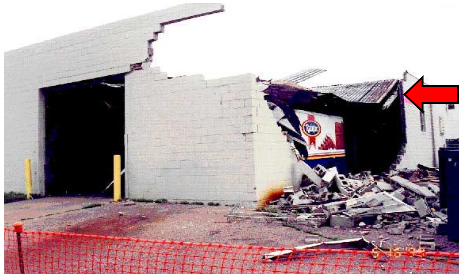
FIGURE 5-26: Failure of roof and walls on structure due to increased loads caused by initial failure of garage door, Wichita, Kansas.
