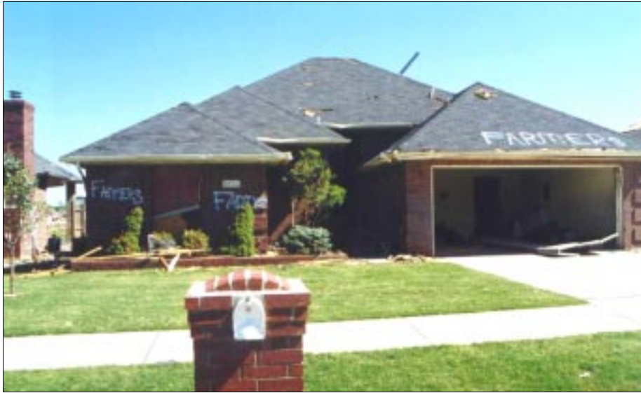
FIGURE 4-23: A view of home G with a garage door that failed due to positive or inward acting wind loads.
