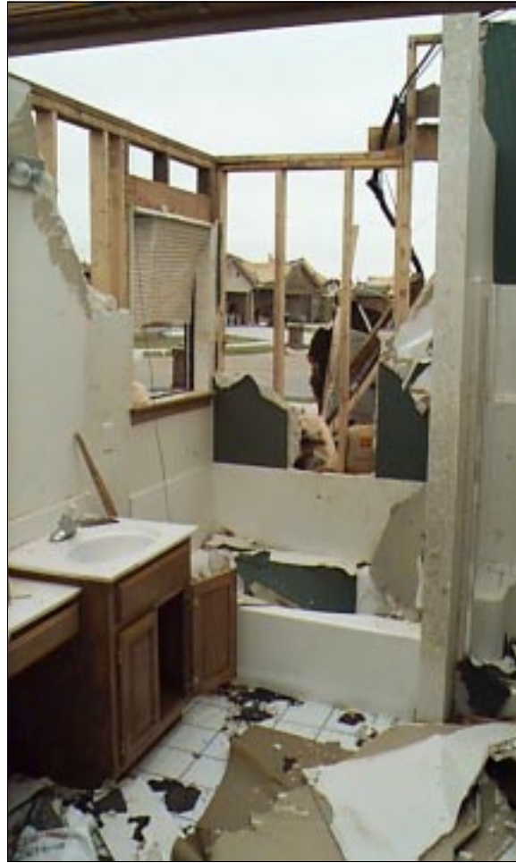
FIGURE 6-26: This bathroom was on an exterior wall and had a window. It was not a safe refuge.
