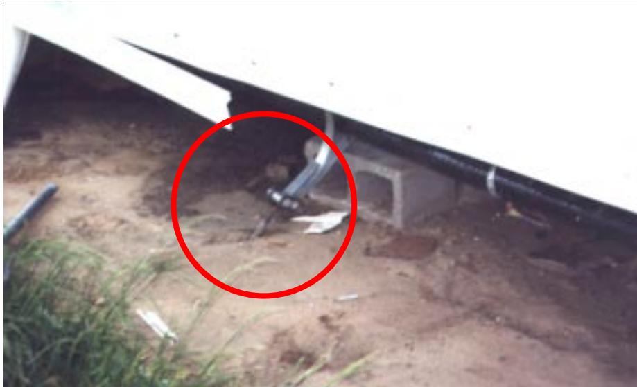
Figure 4-52: Anchor of manufactured home bent and pulled up from soil. This home in Wichita, Kansas, was located within the inflow area of a severe tornado.
