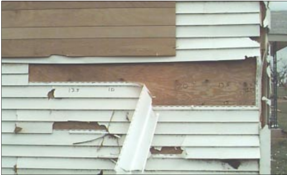
FIGURE 4-17: Some pieces of vinyl siding were blown off and in other areas the siding was torn away by missiles. The home was located along the periphery of a violent tornado in Mullhall, Oklahoma.
