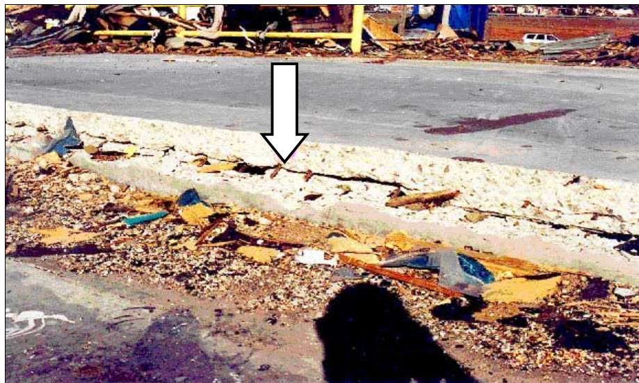
FIGURE 5-16: Failure of tilt-up concrete wall in Del City, Oklahoma, hit by inflow winds of a violent tornado.
