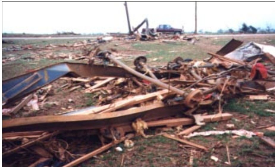
FIGURE 4-50: Strap anchoring failure most likely led to the displacement of this chassis, Bridge Creek, Oklahoma.
