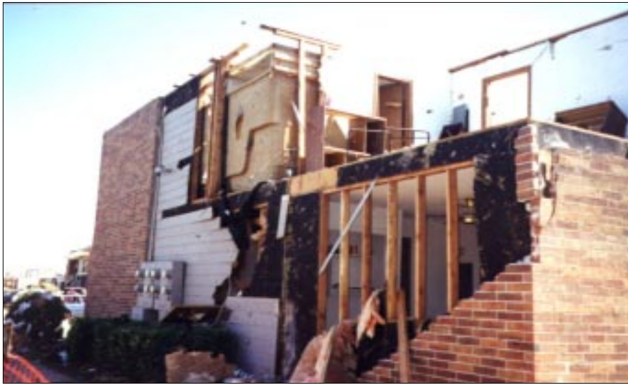
FIGURE 4-11: Stud-wall and sole-plate-to-floor failure on a second story wall. This multi-family residence in Wichita, Kansas, was located approximately a few hundred feet from the vortex of a violent tornado and was exposed to inflow winds.
