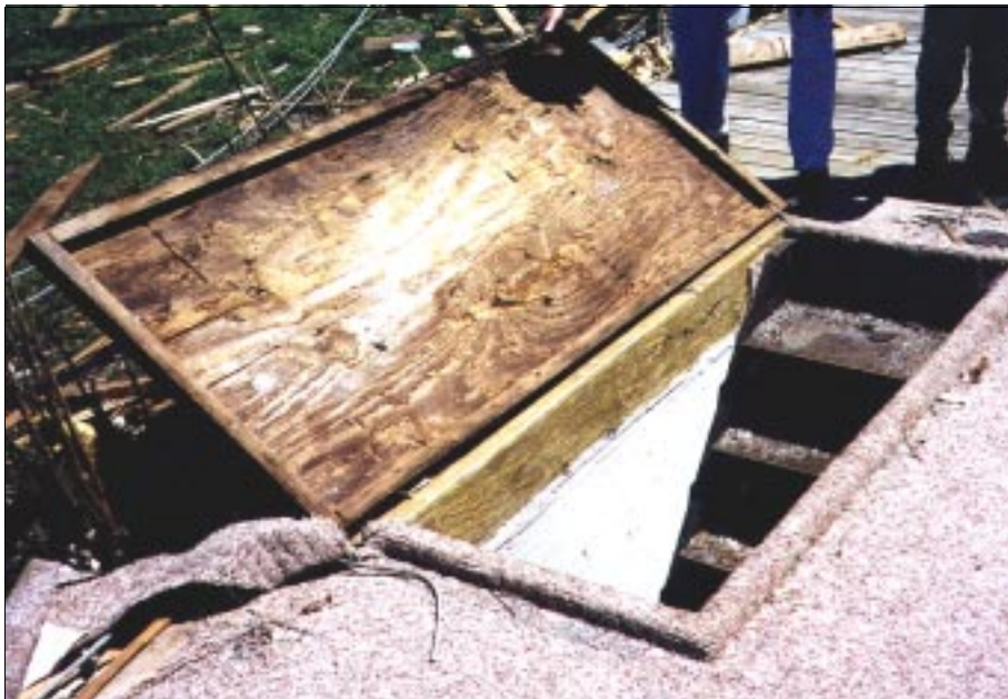
FIGURE 6-12: Door to underground shelter with rotting wood and corroded hinges.
