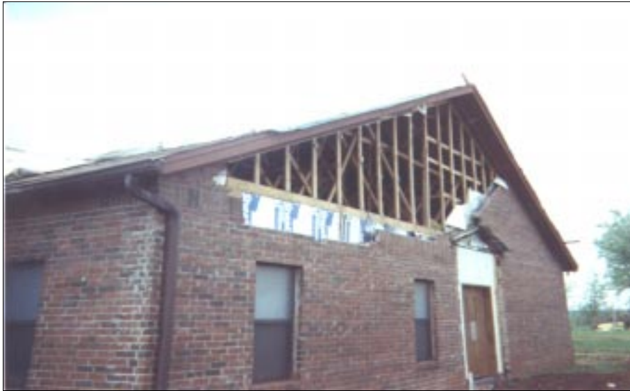
FIGURE 3-6: Failure of this gable wall section was due to wind suction forces of the leeward wall. This house was on the outer edge of a violent tornado path.
