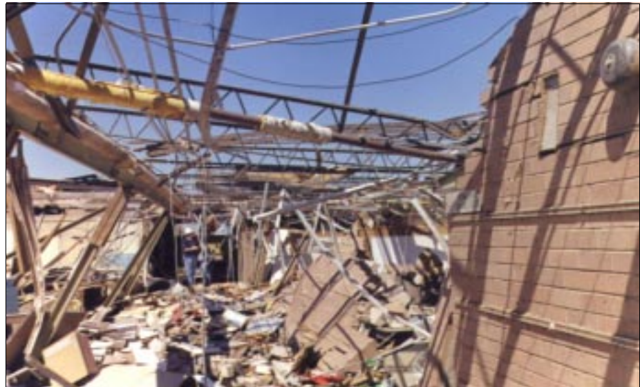
FIGURE 6-32: Kelly Elementary School, Moore, Oklahoma, place of refuge - double loaded corridor with clerestory windows. These interior corridor walls had brick masonry up to a height of approximately 7 feet. Glass extended from the top of the masonry to the top of the wall.
