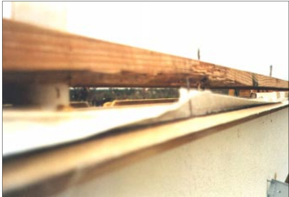
FIGURE 4-8: Failure of a double top-plate. The uplift of the roof truss previously attached to this double top-plate caused separation of the two members that comprise this top-plate.
