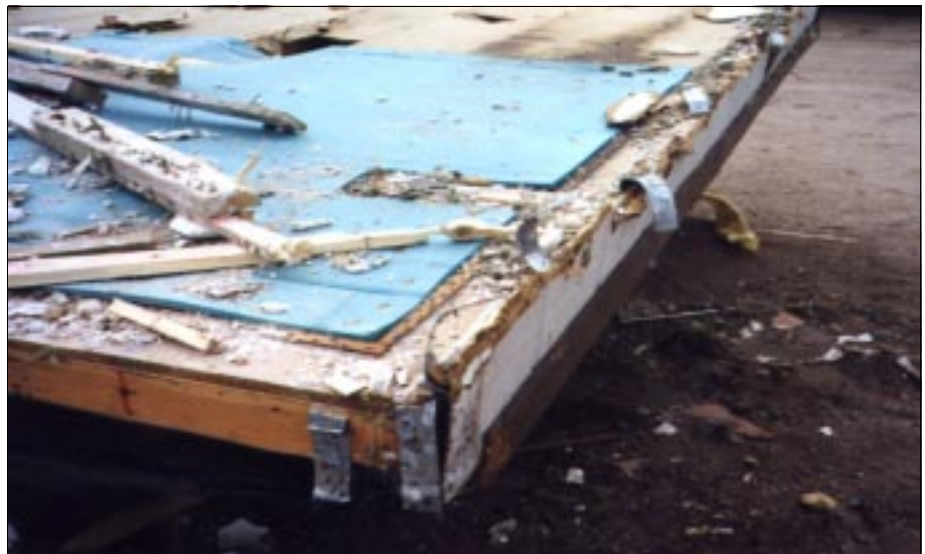
FIGURE 4-57: A close up of the manufactured home floor and chassis after it was removed from the permanent foundation in Figure 4-56.
