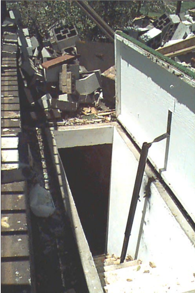
FIGURE 6-20: This below ground shelter is susceptible to water runoff.
