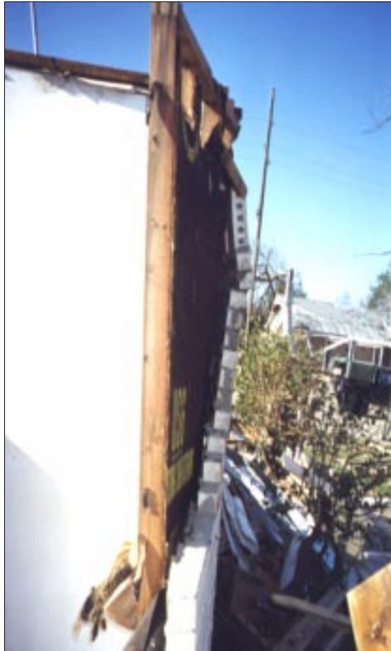
FIGURE 4-36: Failure of masonry veneer wall, Del City, Oklahoma.
