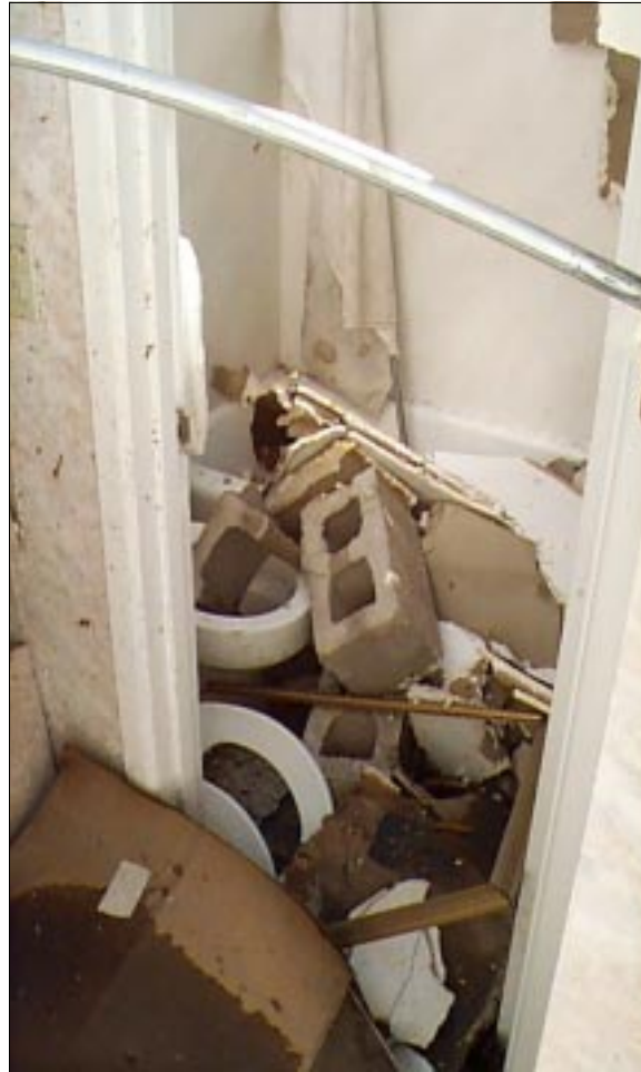
FIGURE 6-36: The roof and ceiling over this interior bathroom blew off. CMU from a firewall a few feet away blew into the bathroom, which was located on a motel's second floor in Mid West City, Oklahoma. This bathroom was not a safe refuge when impacted by the vortex of a severe tornado.
