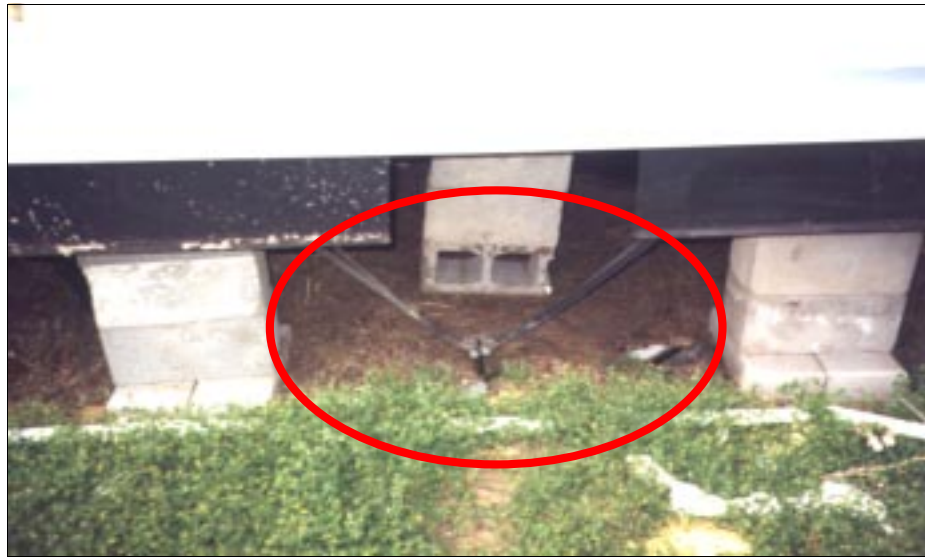
FIGURE 4-60: View of anchor strap and attachment indicating some lateral shifting of a manufactured home located along the periphery of a violent tornado, Wichita, Kansas.
