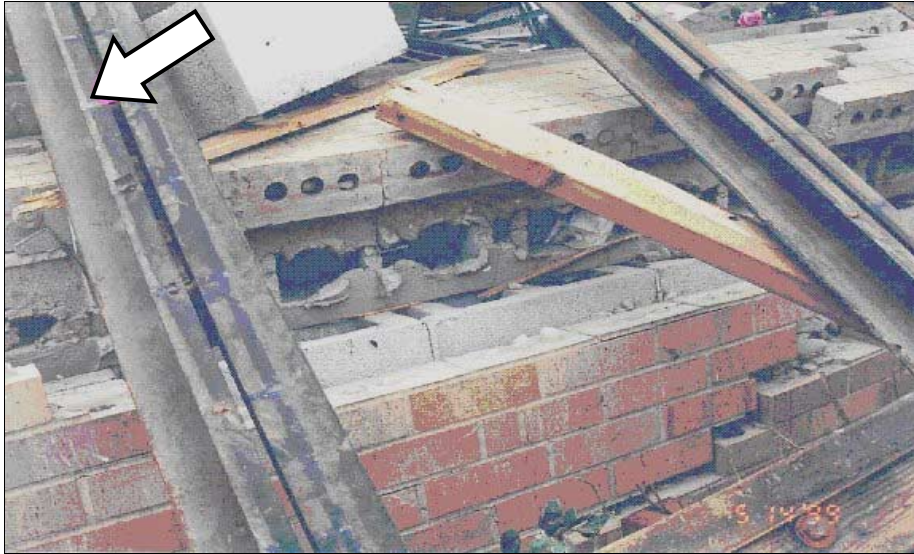
FIGURE 5-4: Failed structure showing broken deck welds, and no effective vertical reinforcement. Kelly Elementary School, Moore, Oklahoma, hit by vortex of violent tornado.
