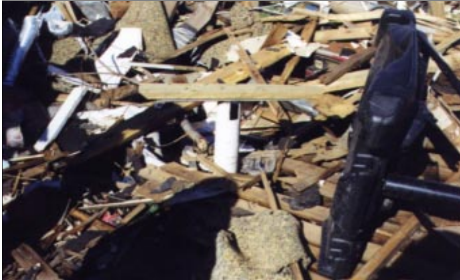
FIGURE 6-18: Heavy gauge ventilation pipe for a below ground shelter in Oklahoma withstood considerable debris impact.
