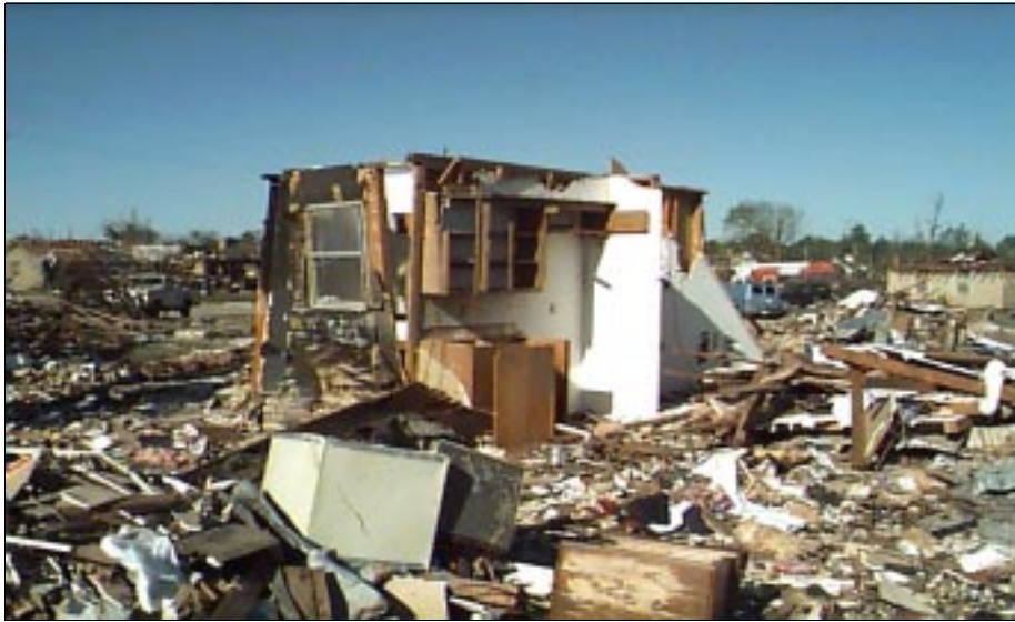
FIGURE 6-22: Interior core of house remains, consisting of a bathroom, closets and a wall with kitchen cabinets after being struck by a severe tornado.
