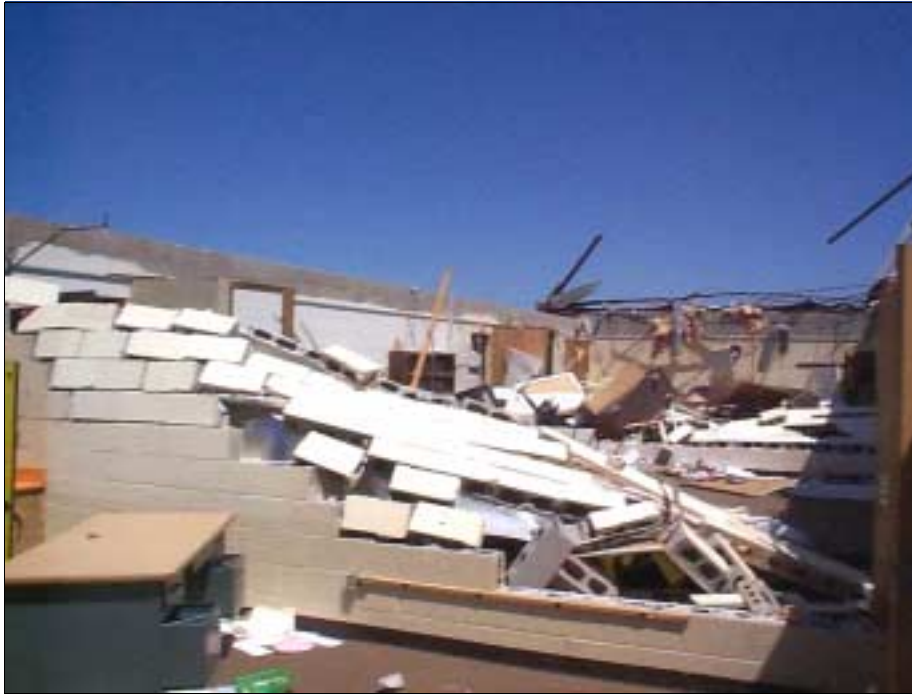
Figure 5-20: Damage to interior and exterior unreinforced masonry walls when bond beam failed at Kelly Elementary School in Moore, Oklahoma. The school was struck by the vortex of a violent tornado.
