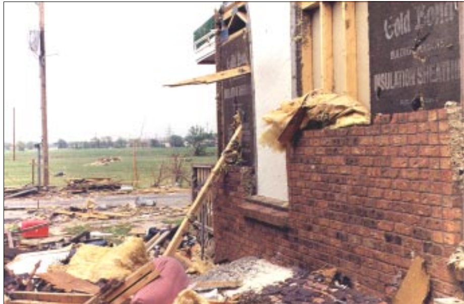
FIGURE 4-44: Failure of masonry veneer at a multi-family housing unit in Wichita, Kansas. This building experienced inflow winds from a severe tornado.
