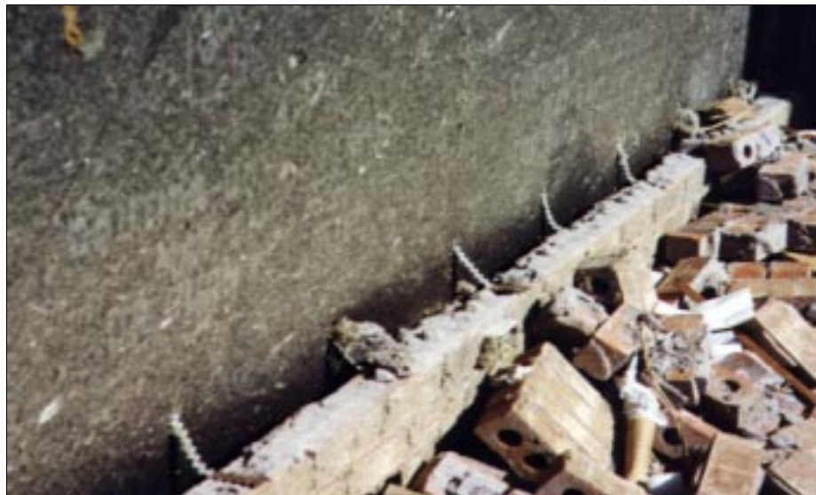
FIGURE 4-33: Failure of masonry veneer wall, close-up view, Moore, Oklahoma. This home was located along the periphery of a violent tornado.
