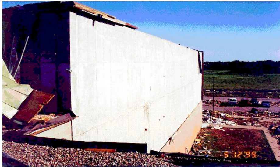
FIGURE 5-15: Exterior view of an undamaged reinforced concrete wall, Westmoore High School, Moore, Oklahoma, hit by inflow winds of a violent tornado. Note: decorative metal wall covering was peeled from this wall.
