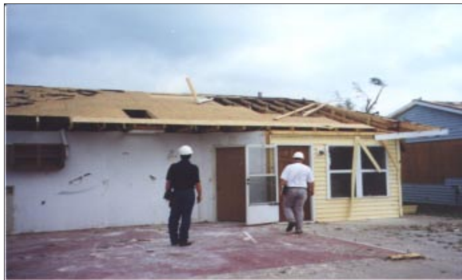
FIGURE 4-4: Although roof sheathing was lost at this Wichita, Kansas, home code requirements of staggering joints in sheathing applications was observed. This house experienced inflow winds from a severe tornado.
