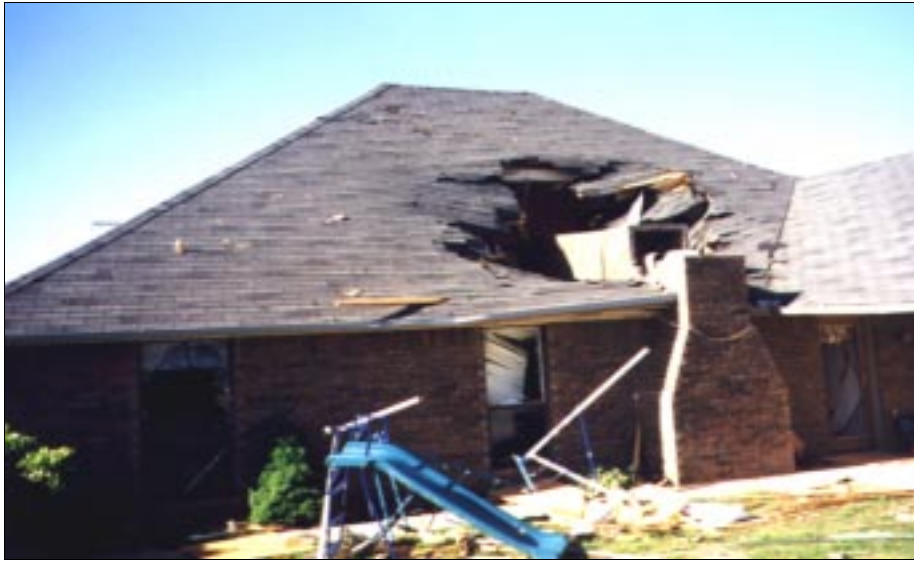
FIGURE 4-42: Failure of brick chimney onto top of home located along the periphery of a violent tornado, Moore, Oklahoma.
