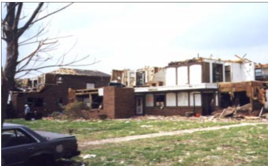
FIGURE 4-43: Failure of masonry veneer.
