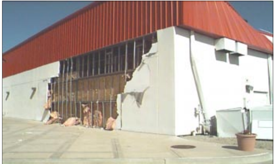
FIGURE 6-34: EIFS wall system torn from metal wall studs.
