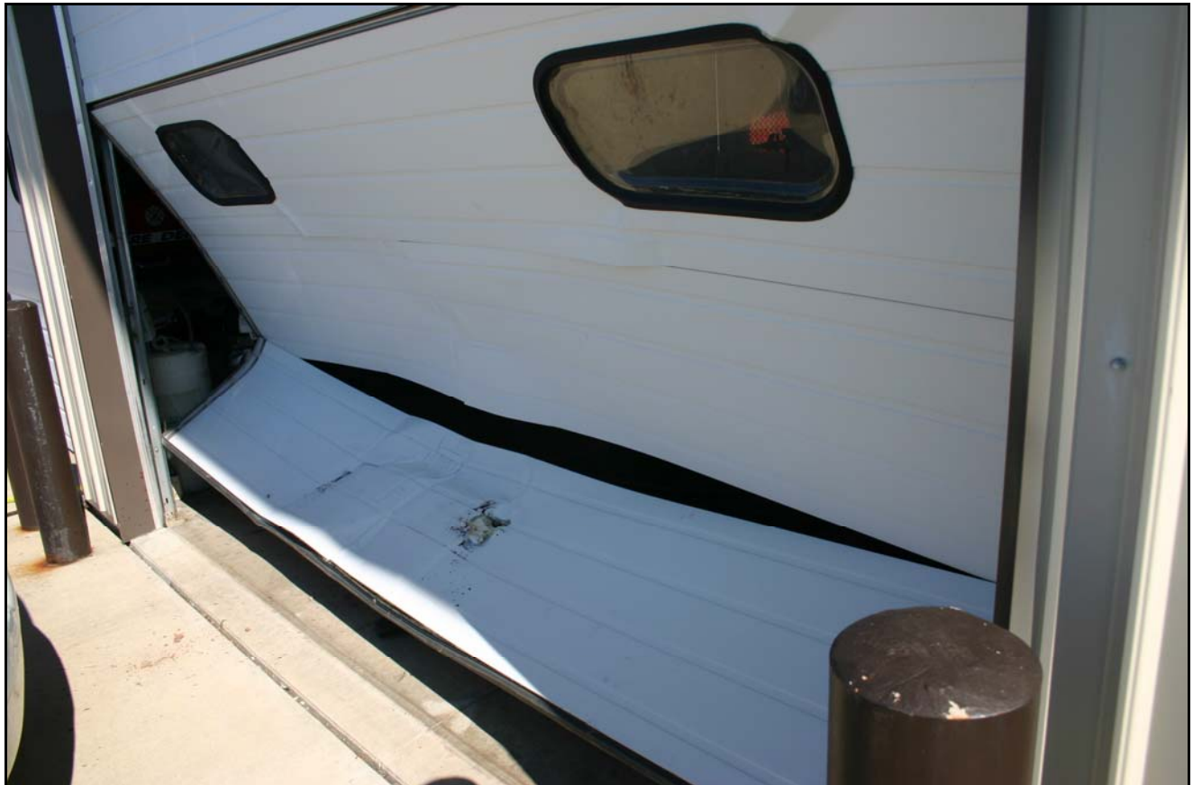
Photo 1. Damage to bay door. (Photo courtesy of Sheriff's Office)
