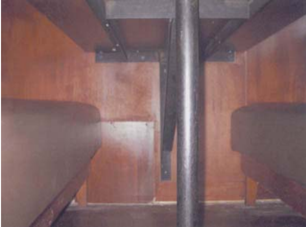
Photograph 2. The origin of the odor (overheated wiring inside the wall).
