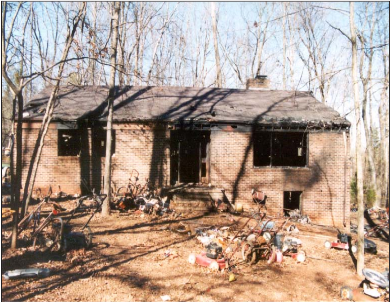
Photo. Front of Structure Involved in Incident (D-Side)
