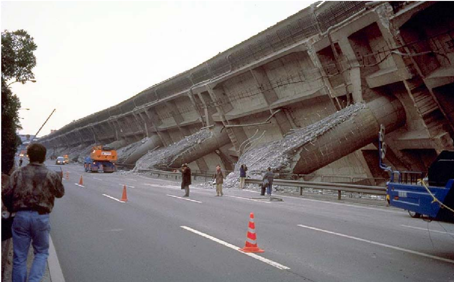
Collapsed Hanshin Highway in Kobe
