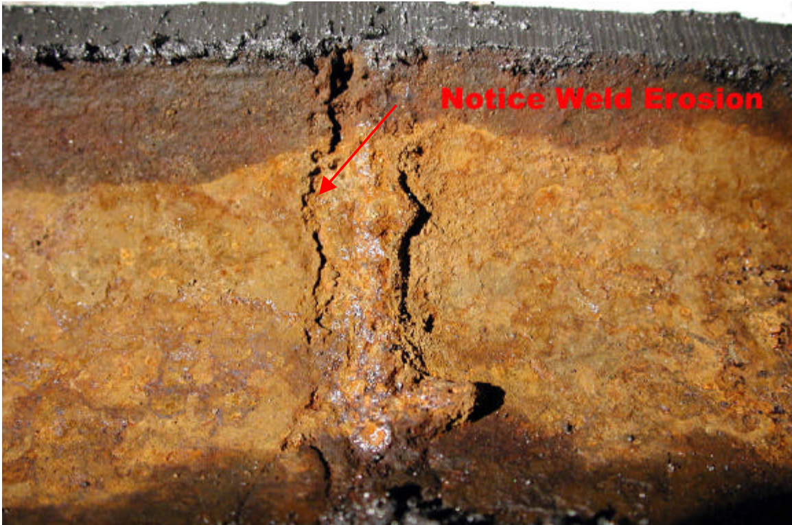
Photos #14 and #15 - Sample Photos from Line 2820
