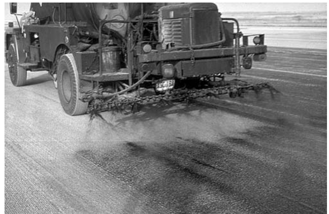
FIGURE 14-8 Improperly adjusted distributor.
