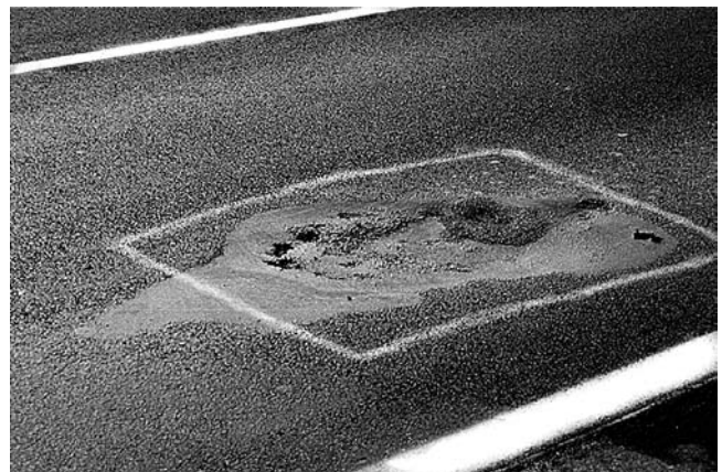
FIGURE 13-7 Pothole caused by overlaying of spilled diesel fuel.
