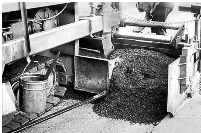
FIGURE 15-22 Buildup of excess mix in front of extended screed.
