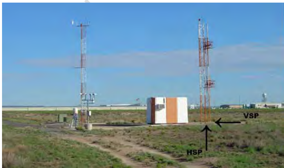
Figure C-6. Typical glideslope installation.
