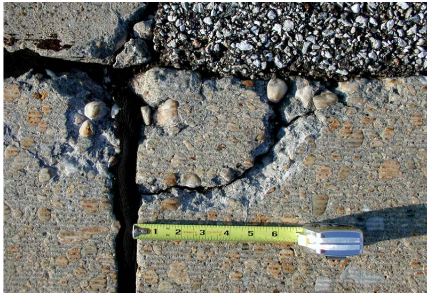
Figure 2-17. Corner spall in another airfield pavement.
