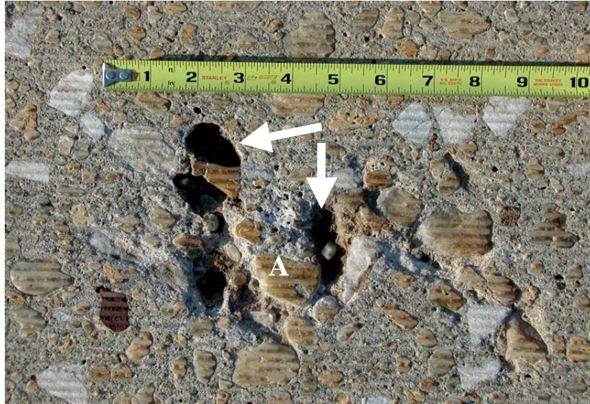
Figure 2-7. Several aggregate particles (A) have been dislodged (→) along with some neighboring paste.
