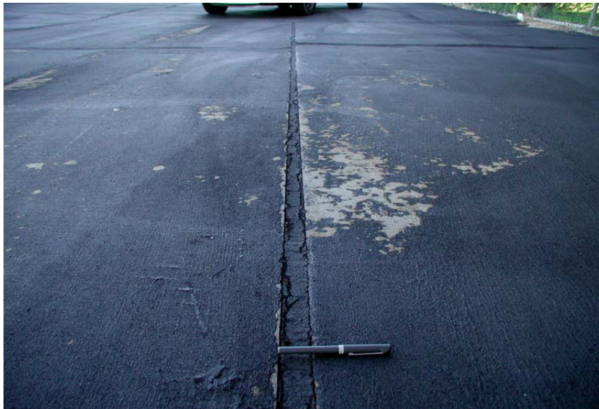
Figure 2-14. Heaving of a slab relative to another
