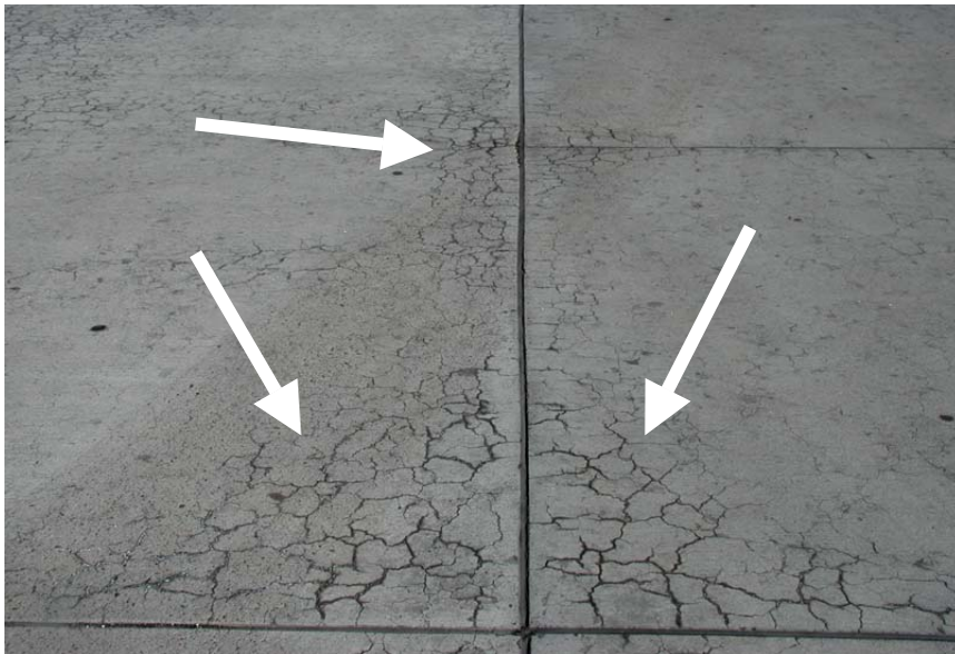
Figure 2-21. Different cracking pattern (→) near the joint of the same pavement section.
