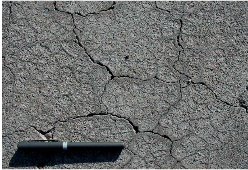
Figure 2-5. Severe map cracking.
