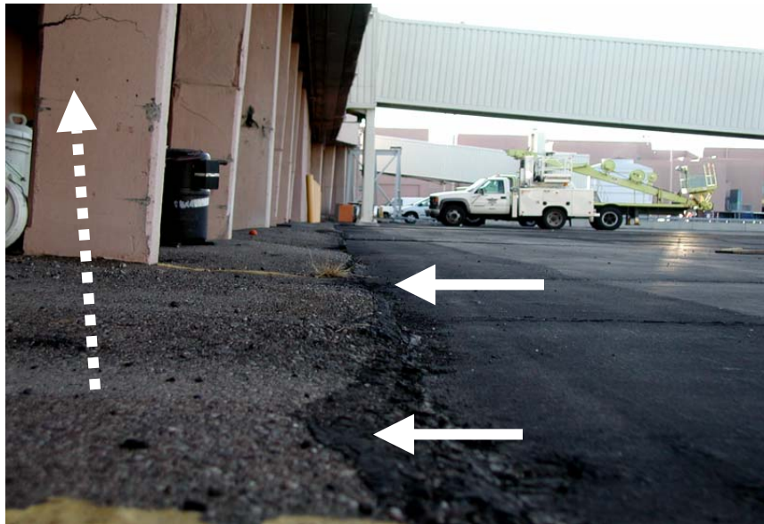
Figure 2-12. Heaving (→) of an asphalt shoulder due to movement of adjoining concrete slab affected by ASR. Movement has been so severe that it has distorted the concrete columns (.....▶) of a neighboring building.
