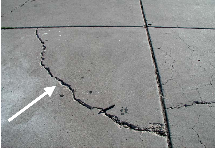
Figure 2-16. Corner break (→) in an airfield pavement.
