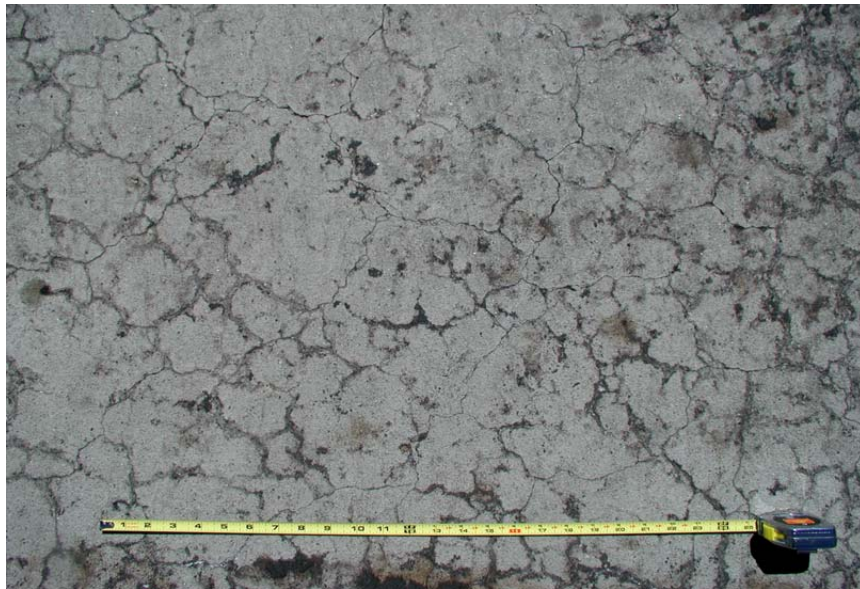
Figure 2-4. Widespread map cracking.
