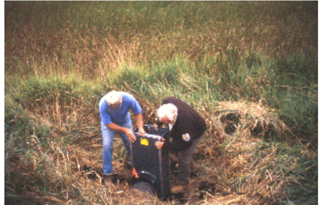
Dave Jacobson, landowner, and Dennis Hall, FWS Engineering Technician, installing a water control structure.
