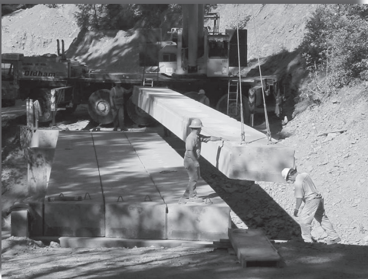
Contractors lower a concrete slab for a new bridge deck across Rock Creek. The bridge replaces an old culvert which hindered fish migration.
