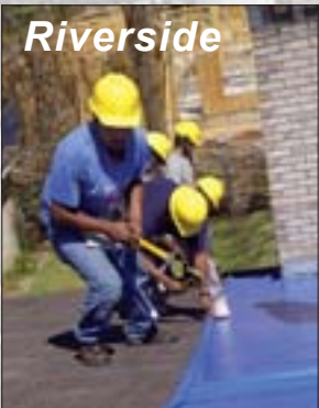
Contractors install a "Blue Roof" on a Florida home damaged by Hurricane Ivan.
