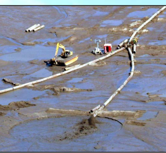
Marsh buggies maneuver the 30-inch diameter pipeline as dredged material is pumped into the disposal site.
