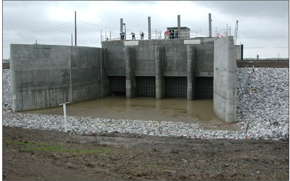
The diversion structure includes the four iron-gated, 14' x 14' box culverts. All four gates should be raised uniformly to maintain a balanced flow of water out of the structure.
