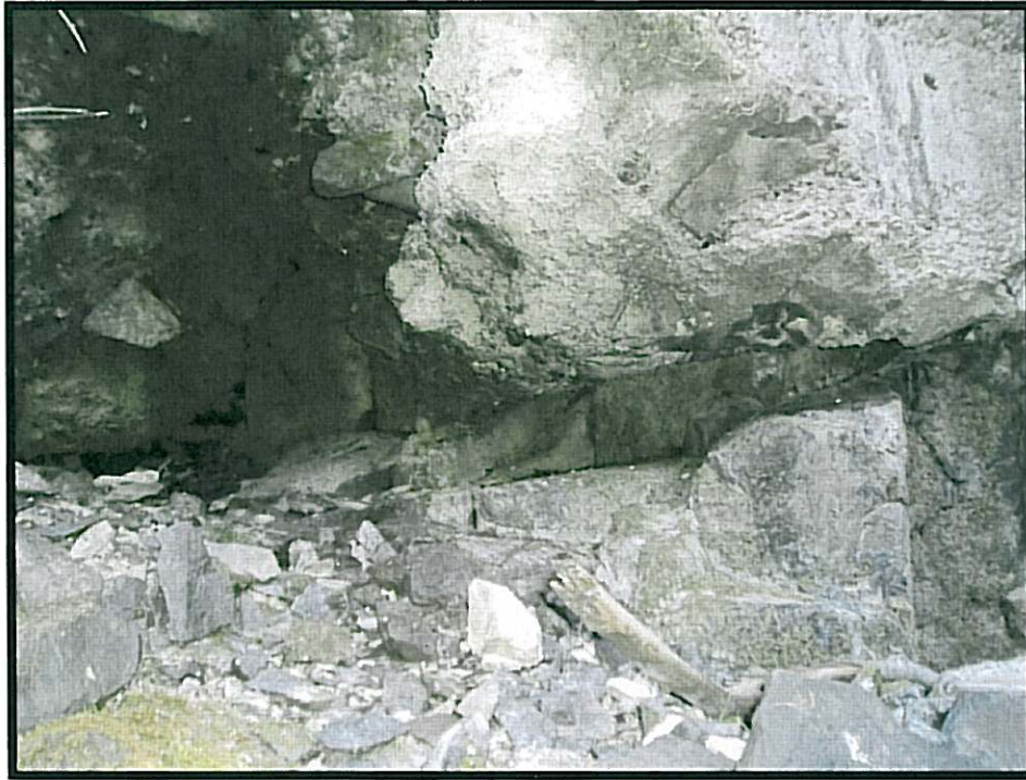
PHOTO 5 – EROSION BEHIND RIGHT ABUTMENT
