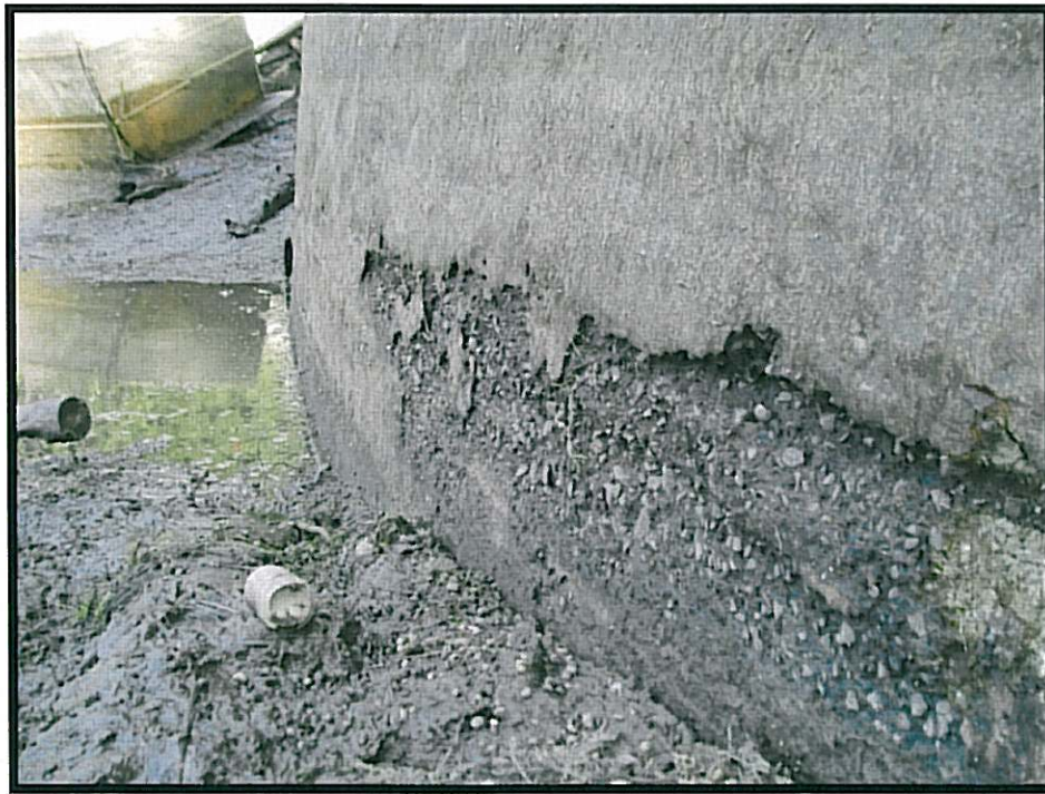
PHOTO 6 – CONCRETE DETERIORATION ON UPSTREAM FACE
