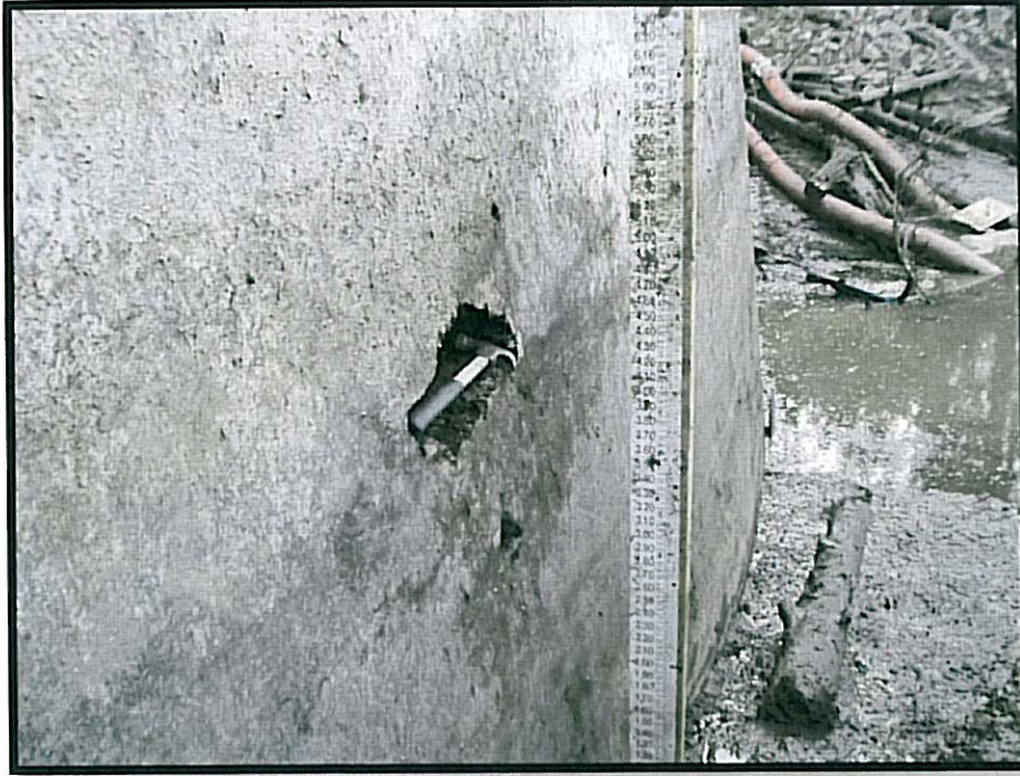
PHOTO 7 – HOLE IN UPSTREAM FACE OF DAM
