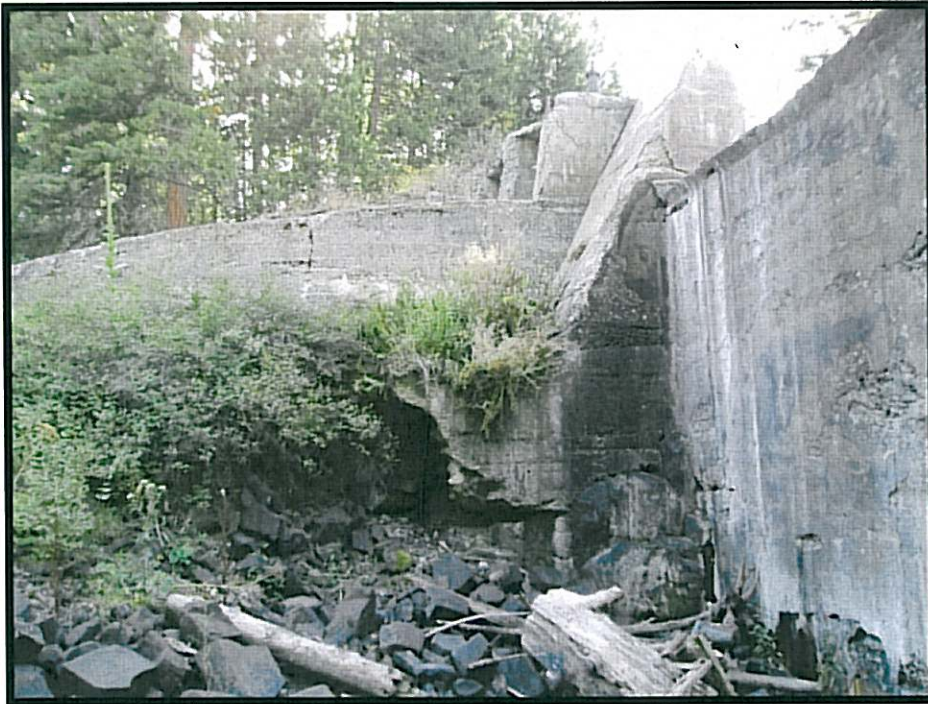
PHOTO 4 – EROSION BEHIND RIGHT ABUTMENT
