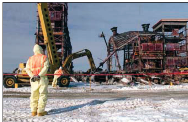
Operating Engineers use Shears to Cut Away Sections of Plant 8 at Fernald
