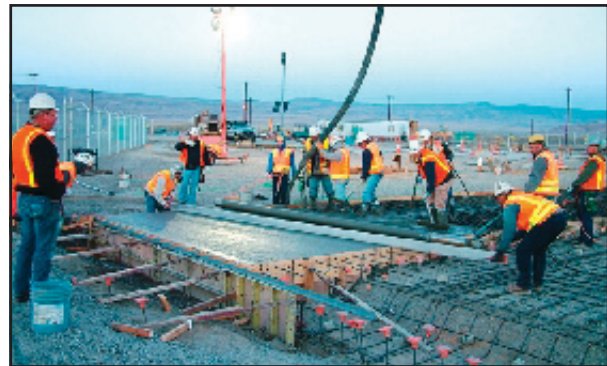
Construction workers completing the concrete work at the Bulk Vitrification Pilot Plant, Hanford.
