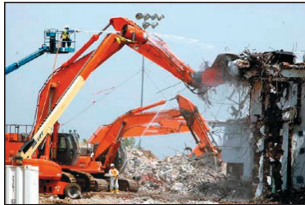
Toppling B371 at Rocky Flats where reinforced concrete walls were up to 4' thick in some areas.
