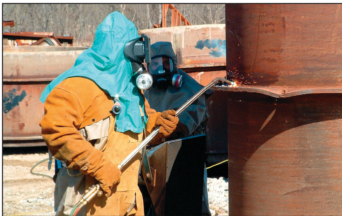
Large Sections of Low Level Radioactively Contaminated Scrap Metal are Sized and Reduced to Fit Into Containers That are Shipped Off-Site for Disposal: Portsmouth Gaseous Diffusion Plant
