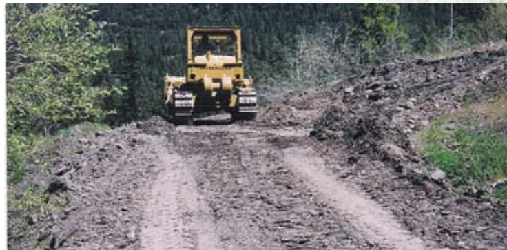
Left unattended, roads will continue to deteriorate with unacceptable consequences.
