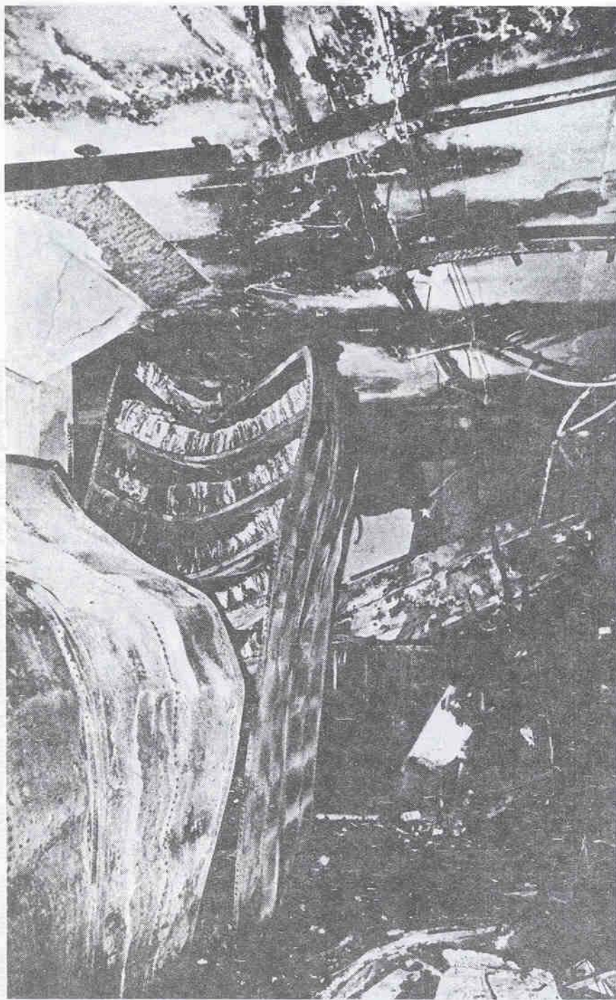
Shelving crushed by the collapsed roof of sixth floor records storage area.
