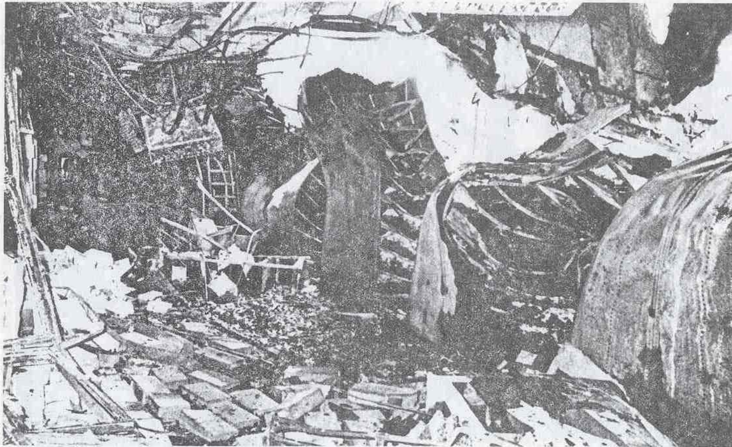
Damaged shelving, broken sections of concrete roof slab, and sky in background.
