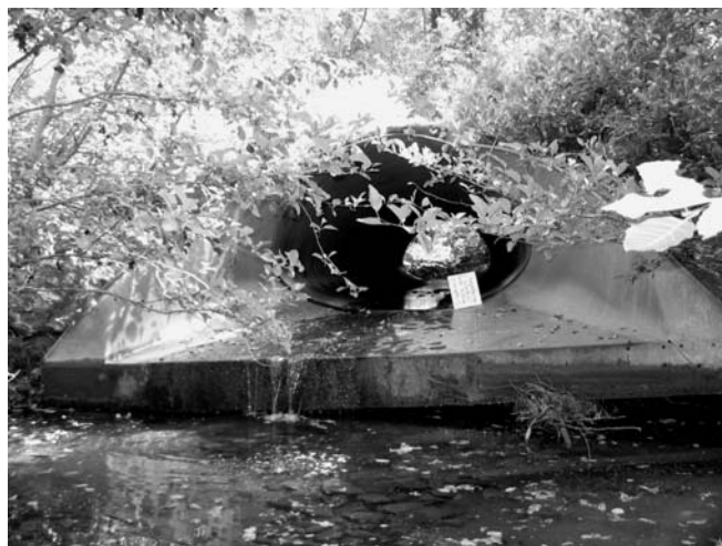
Figure 1-6. Gold Run Creek culvert on road 20N95. This elevated culvert blocks fish from reaching upstream areas, and the unnatural substrate is poor for aquatic insects. Notice that it has also been undermined.
